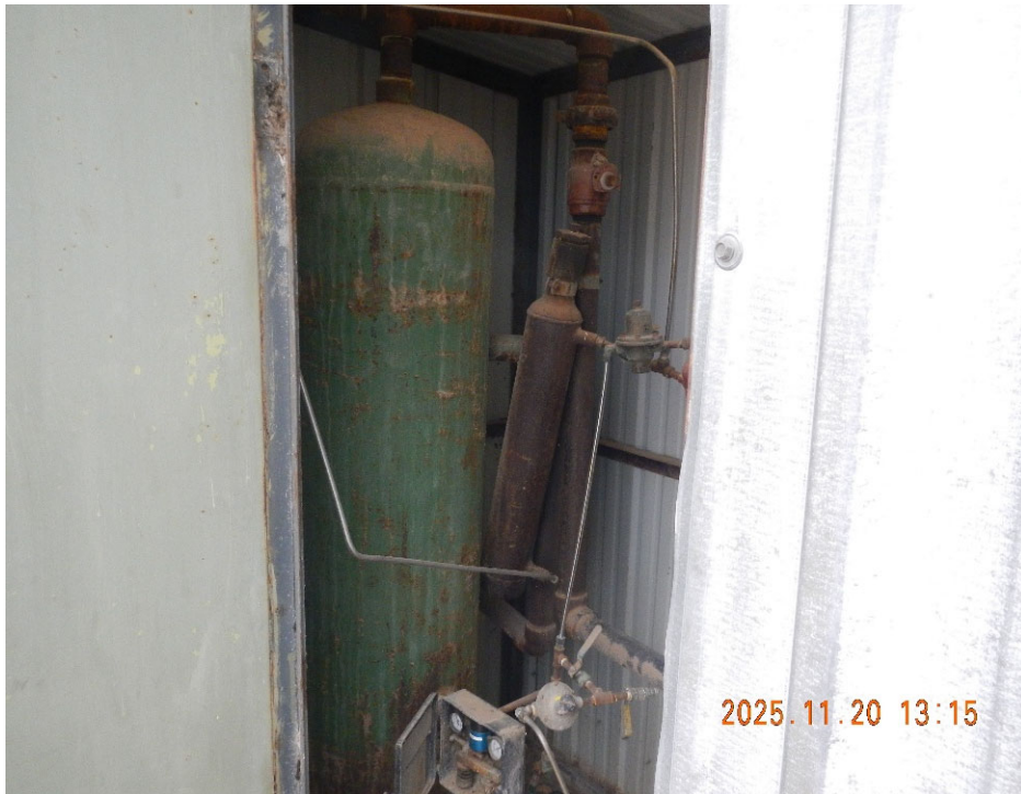
5. Vertical Separator inside Meter Shed.
