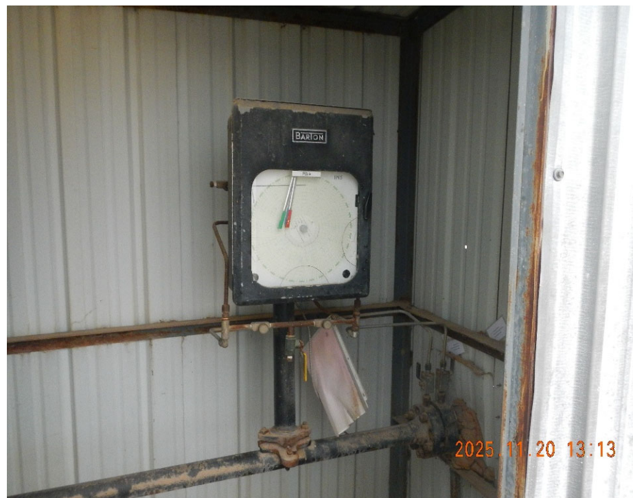
4. Gas Meter inside Meter Shed.
