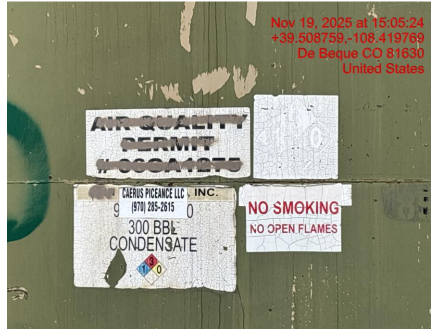
Tank Labels Missing Required Information – Photo #01609
