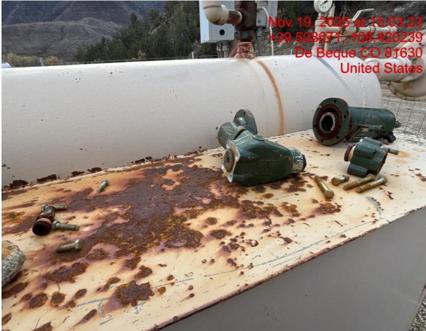
Stored Supplies on Separator – Photo #01605
