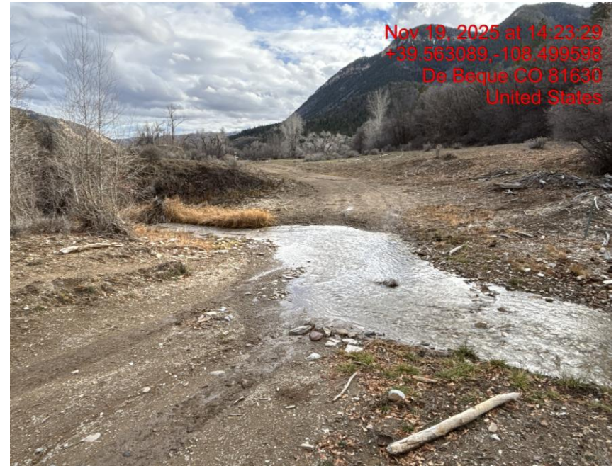
No Erosion Controls Installed at Stream Crossing – Photo #01594
