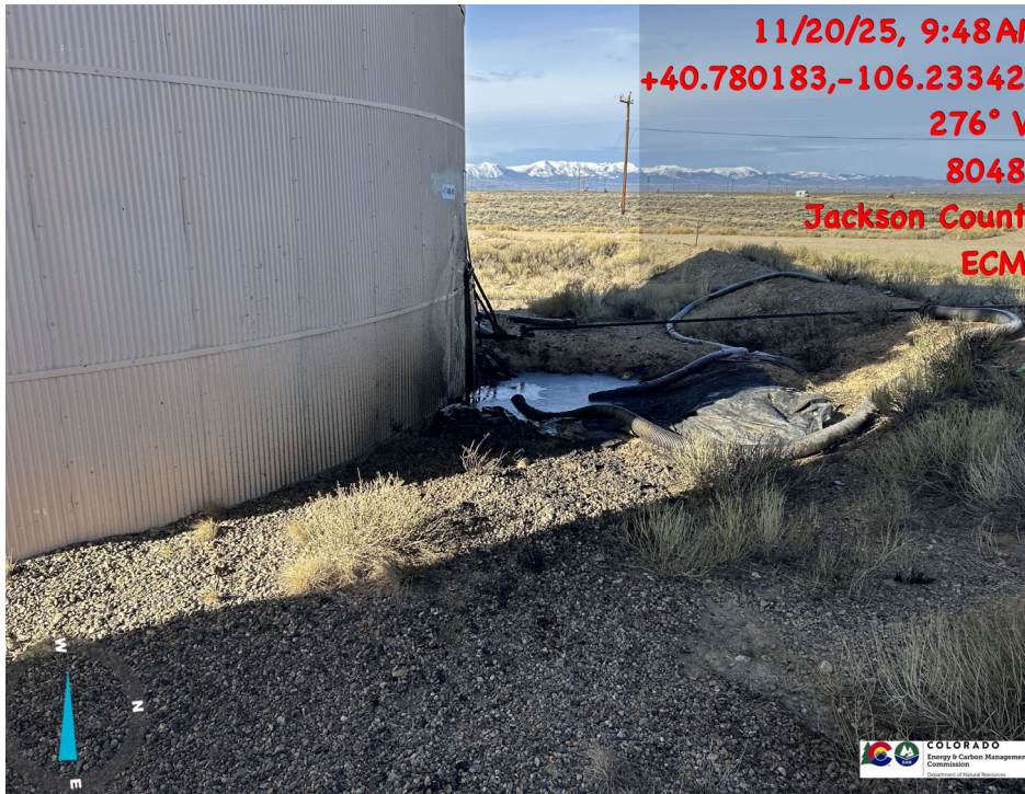
Staining and debris
