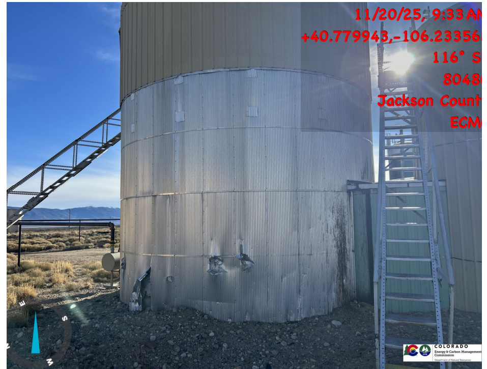
Tank lacks legible labeling and debris
