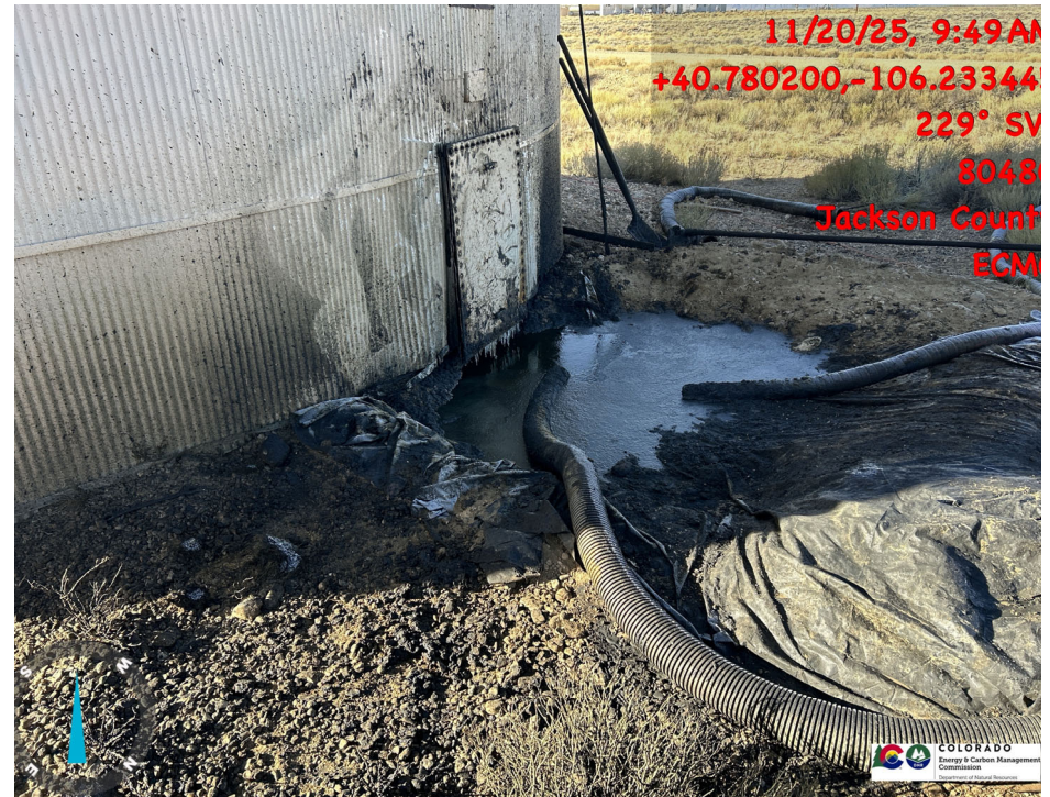
Leaking tank and staining
