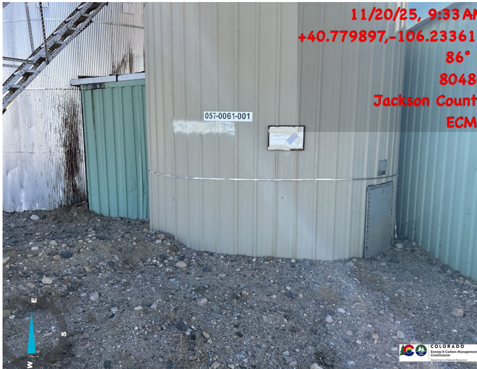
Tank lacks legible labeling and debris
