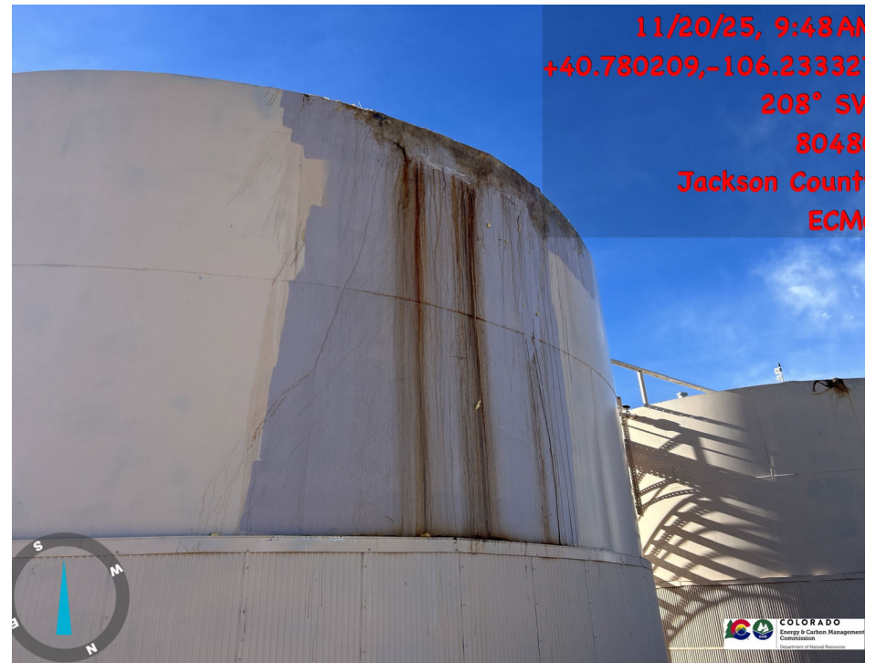
Crack in tank sealed with fiberglass patch
