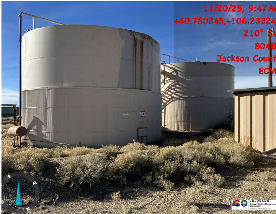
Tank that was leaking emissions
