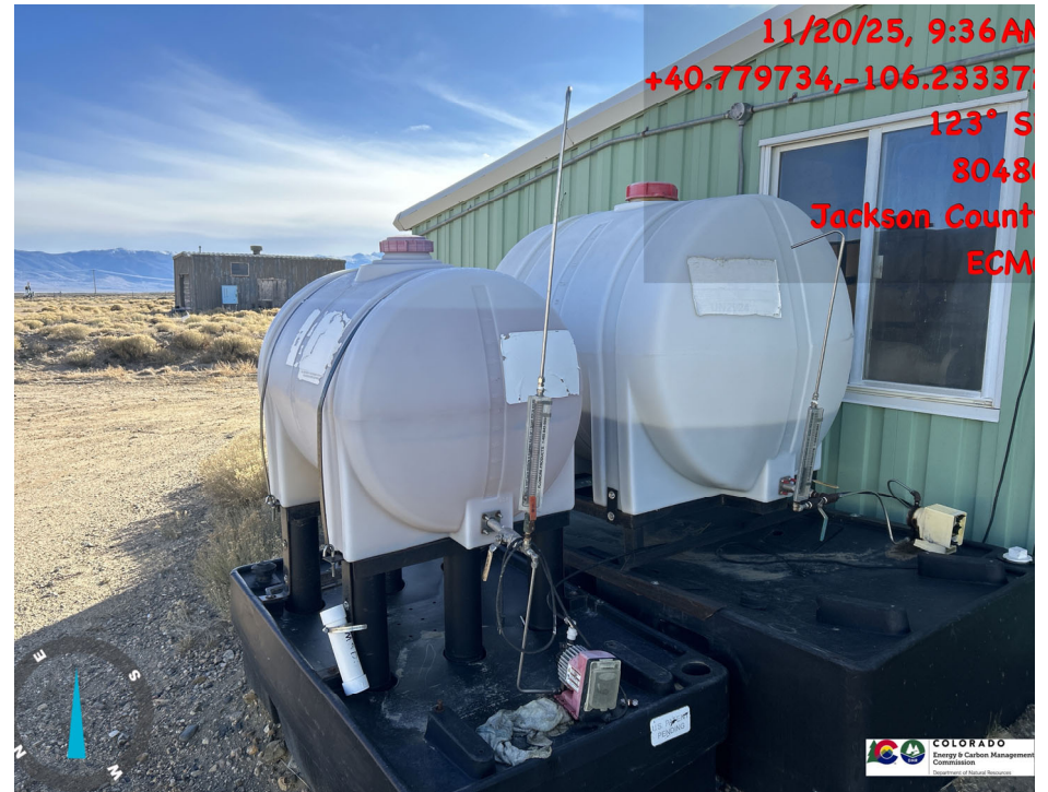
Chemical tanks lacking legible labeling
