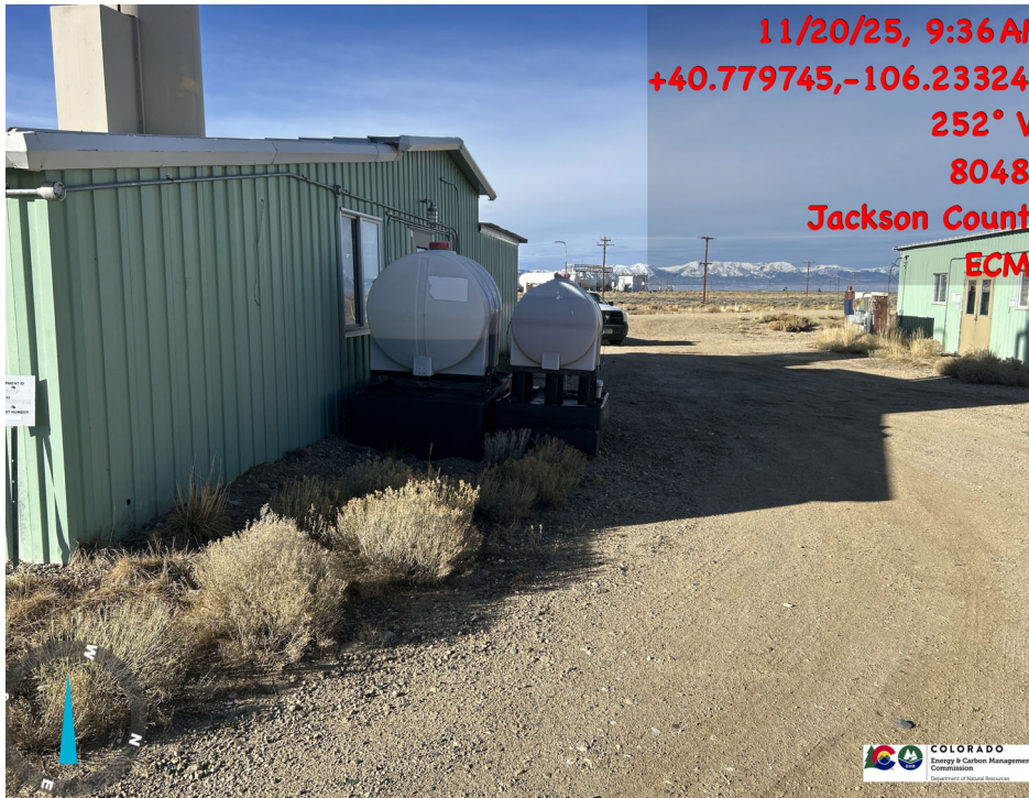
Chemical tanks lacking legible labeling
