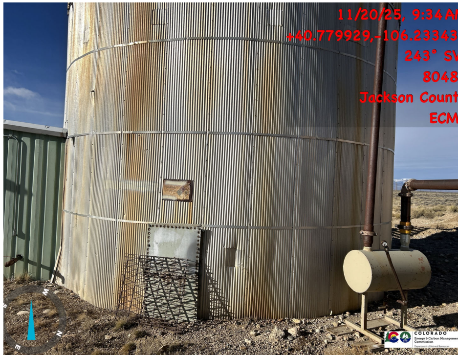
Tank lacks legible labeling and debris
