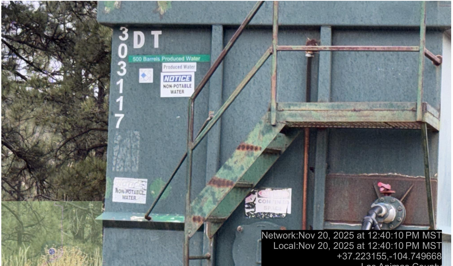
PHOTO 3: INADEQUATE SIGNAGE ON TANK BATTERY
