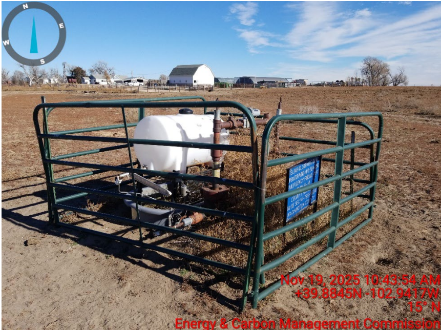
1. Wellhead and chemical tank
