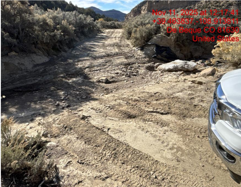
Lease Road Erosion – Photo #01544
