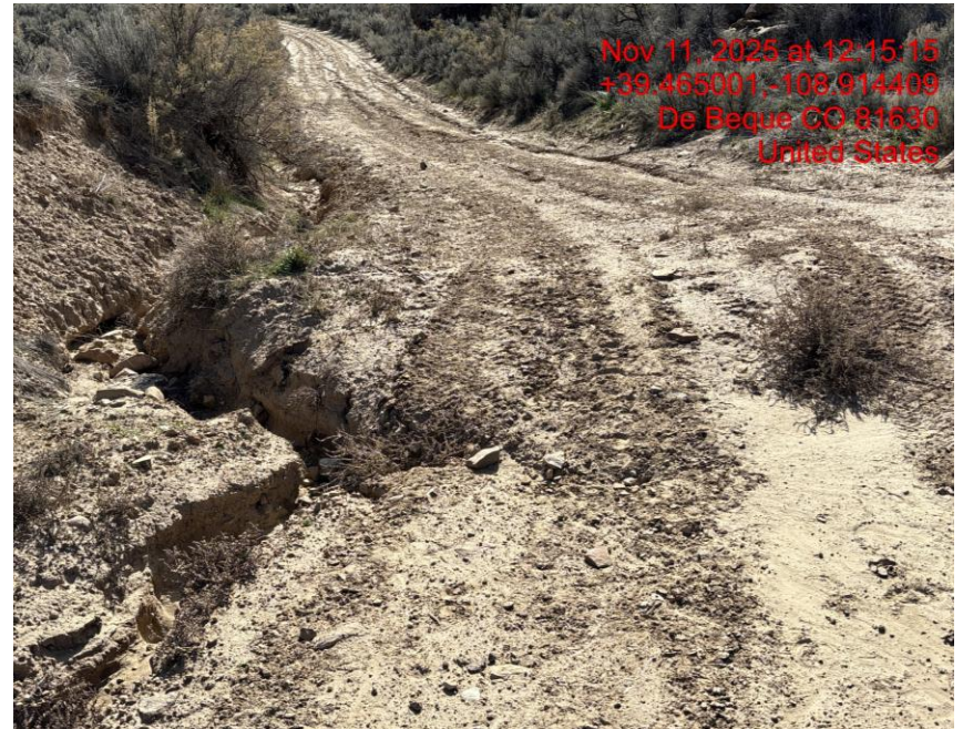
Lease Road Erosion – Photo #01542
