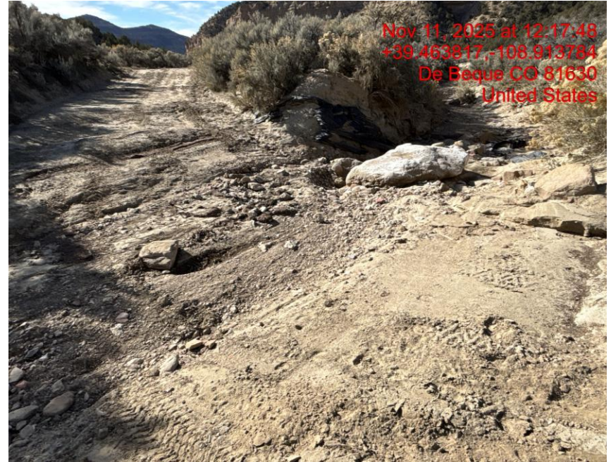
Lease Road Erosion – Photo #01545
