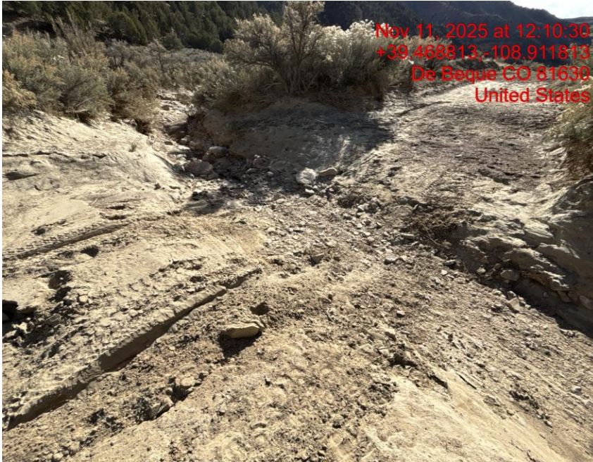
Lease Road Erosion – Photo #01534
