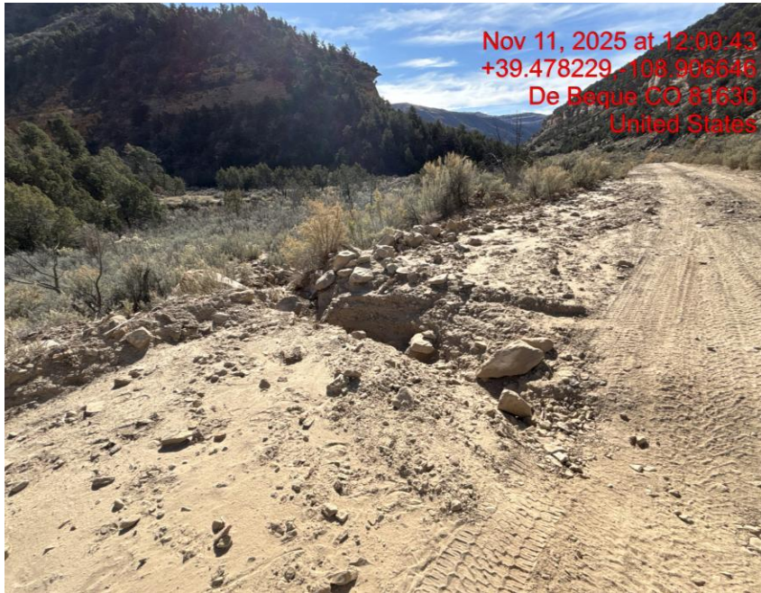
Lease Road Erosion – Photo #01519
