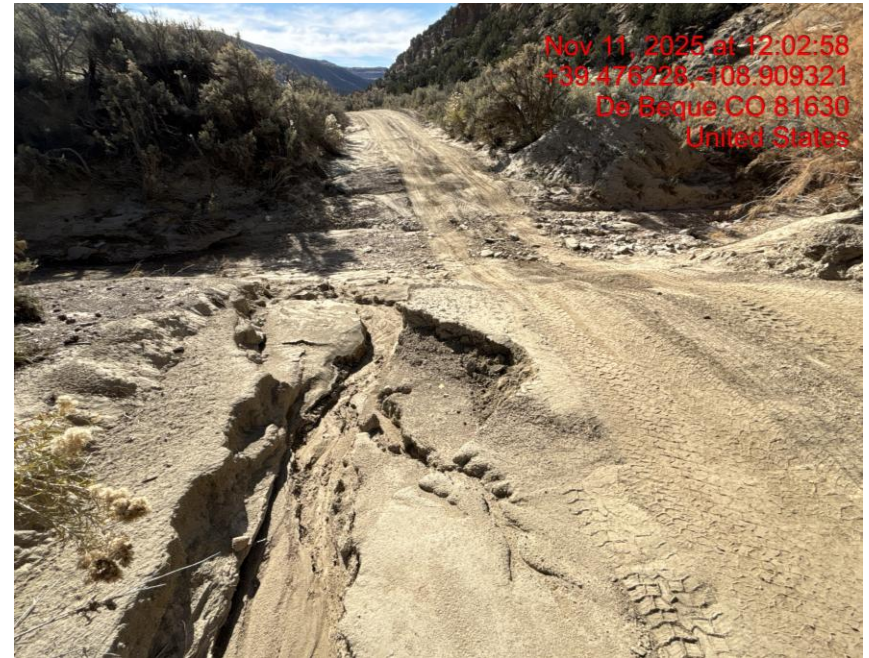
Lease Road Erosion – Photo #01523
