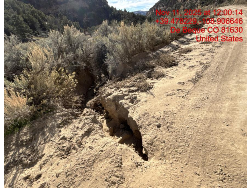
Lease Road Erosion – Photo #01518
