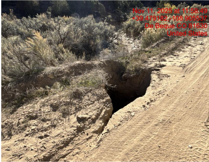
Lease Road Erosion – Photo #01517
