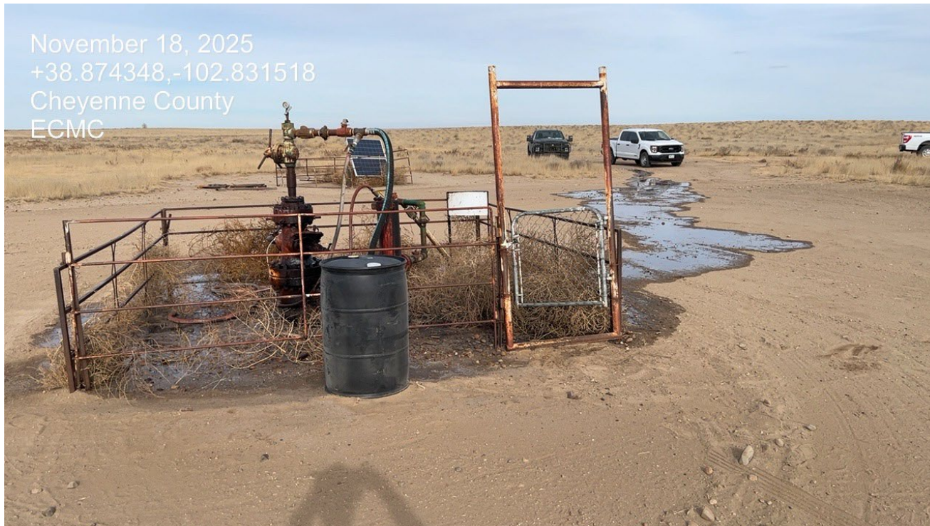
Photo 6. Facing to the northeast at the wellhead. The pumper arrived onsite to turn the valve and stop the leak.
