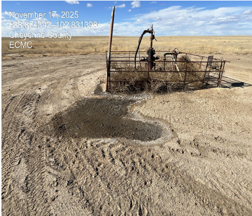
Photo 7. Inspection the day before observed a small spill had occurred at the wellhead.
