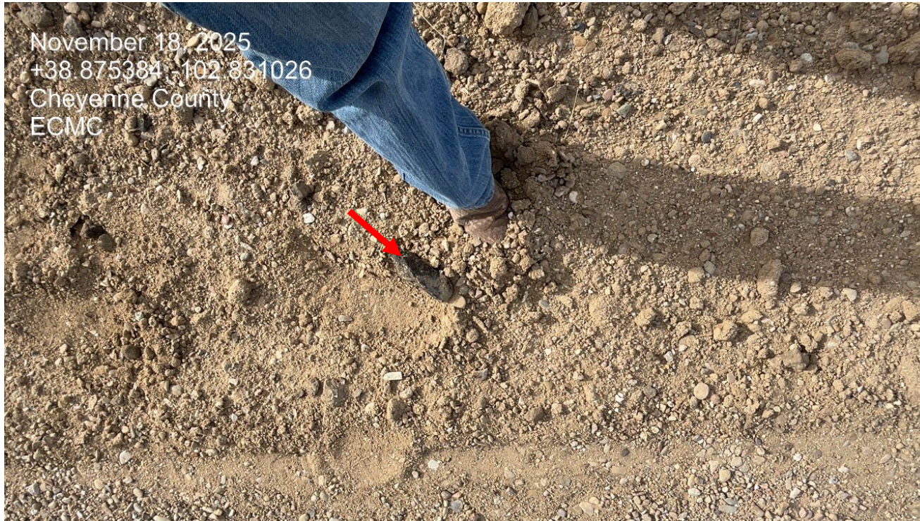
Photo 3. There are chunks of asphalt from material brought in to build up the road. Also material where inspectors foot is placed is loose and needs to be graded and compacted.
