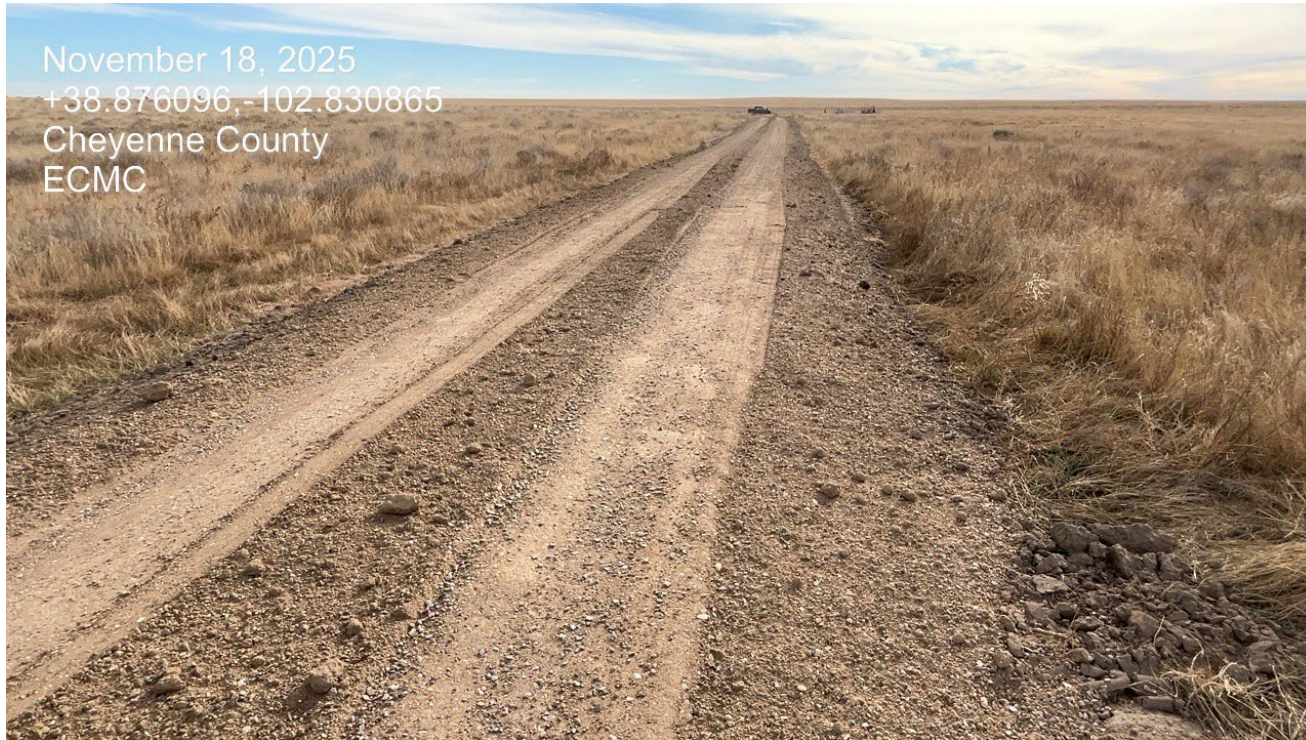
Photo 2. Facing south along the access road. There has been road base material spread along the road where road degradation had occurred.
