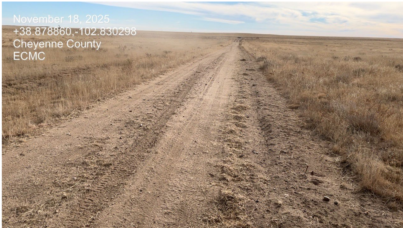
Photo 1. Facing south along the access road. This area was graded with loose soil material from the roadside. The adjacent roadside soils should not be graded, causing the road to widen with additional disturbance.
