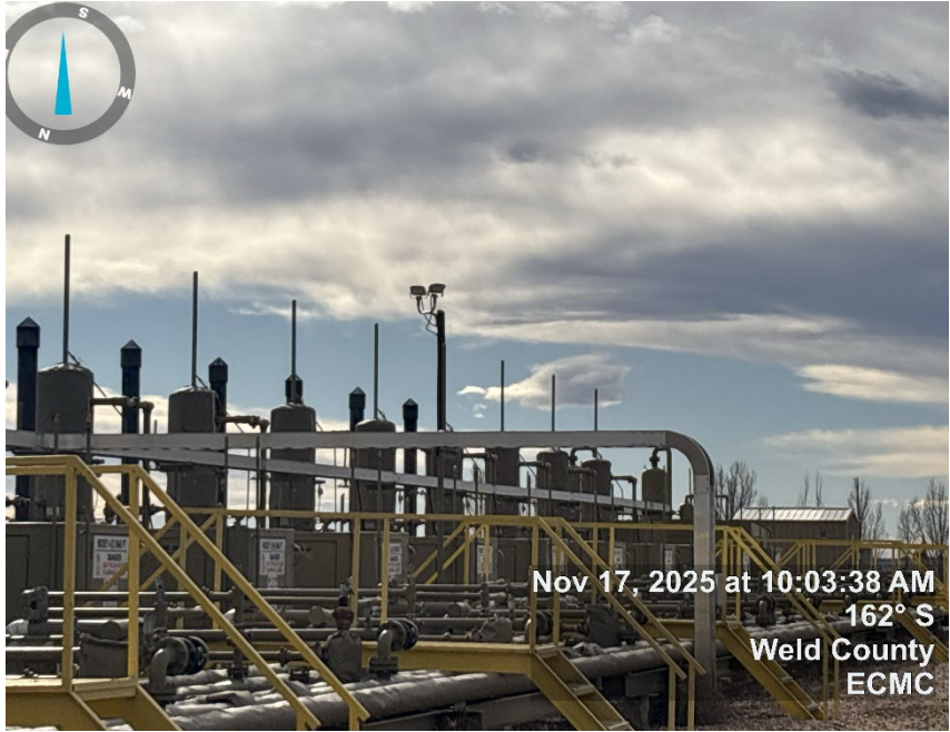
Photo 9: lighting appears to be in down position.
