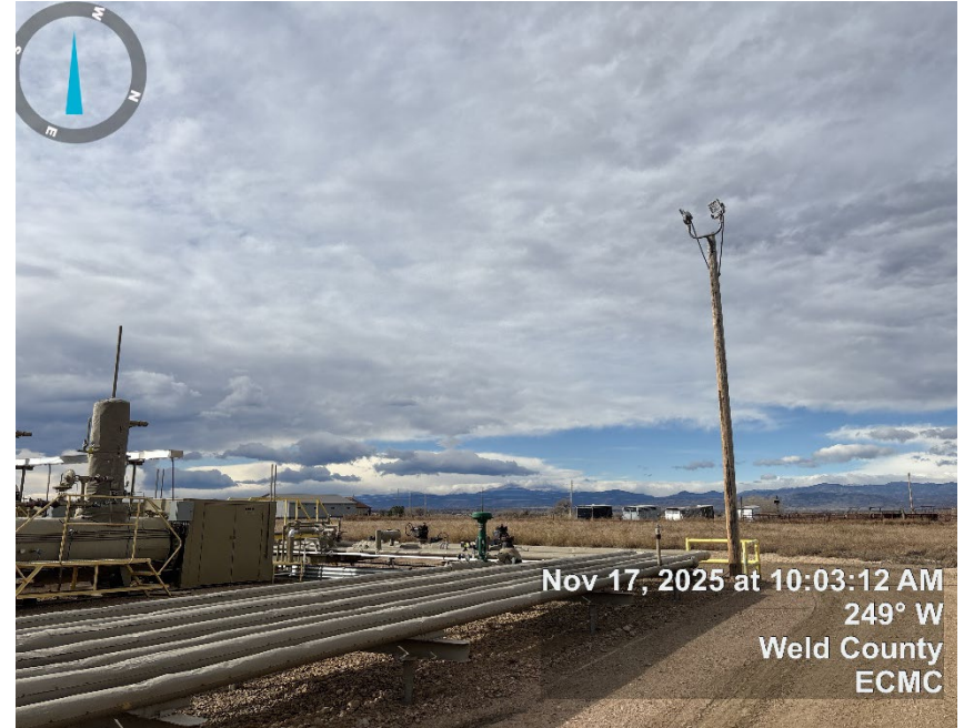
Photo 8: lighting appears to be in down position.
