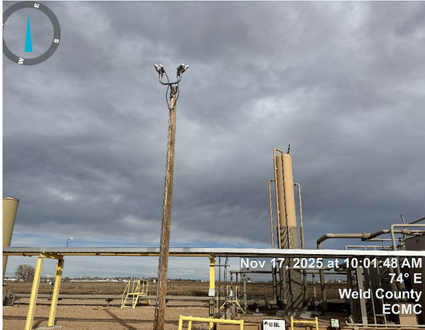
Photo 7: lighting appears to be in down position.
