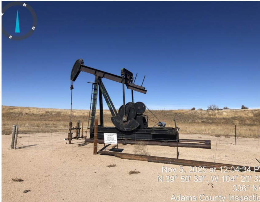
Photo #3 Pump jack & pipe.
