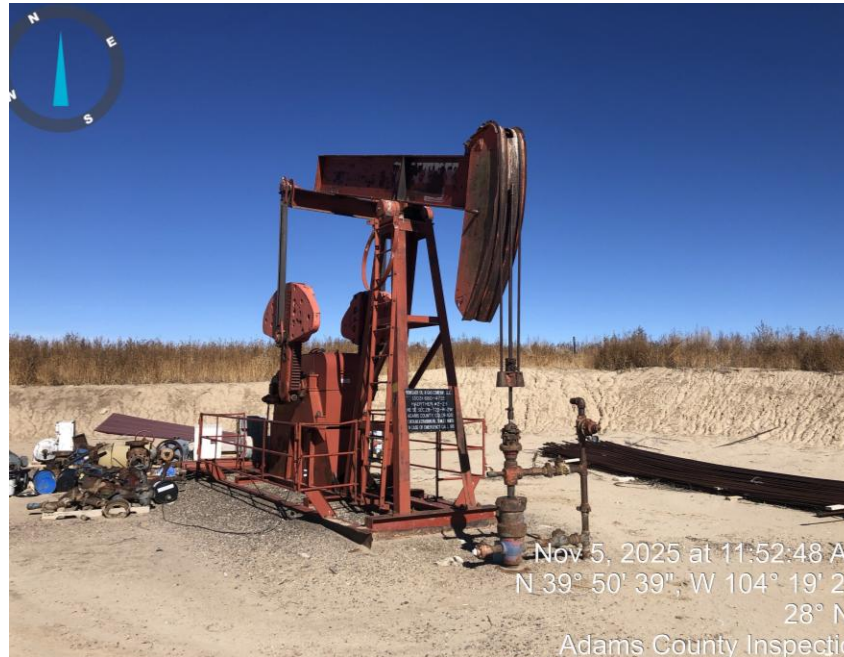
Photo #3 Pump jack & unused equipment.
