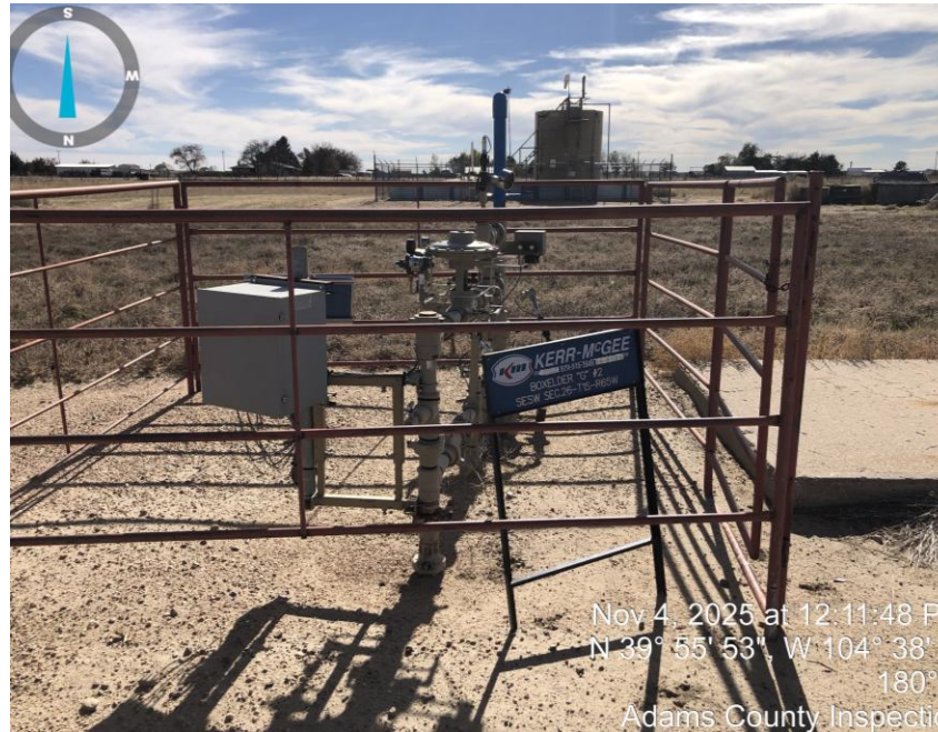
Photo #3 Well head.
