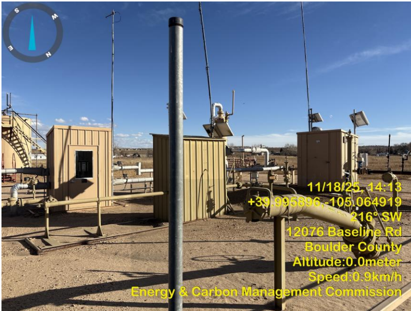
Photo 9 Gas Meter Runs.
