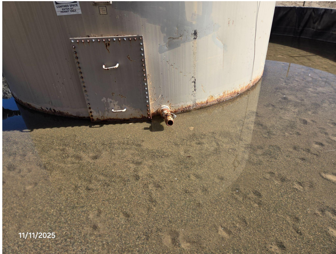
Photo 4: Lines at tank have not been capped or plugged.
