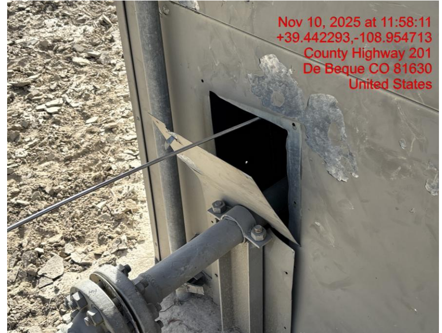
Wildlife Entry Hazard at Gas Meter House – Photo #01498
