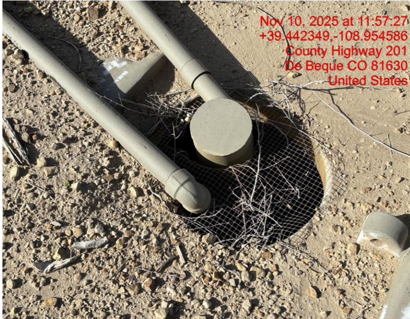
PBV Inlet Open to Stormwater Drainage – Photo #01495
