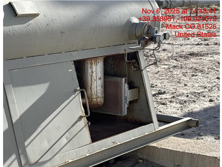
Wildlife Entry Hazard – Photo #01459
