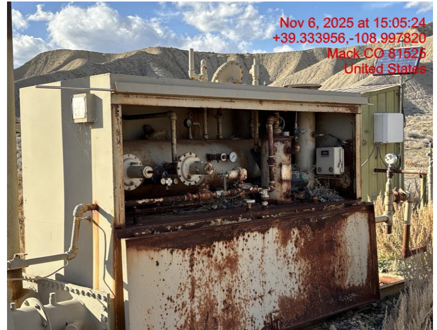
Wildlife Entry Hazard – Photo #01463
