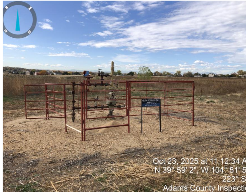
Photo #3 Well head.
