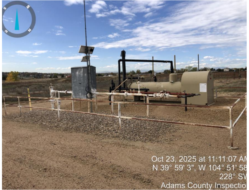
Photo #2 Separator & meter.
