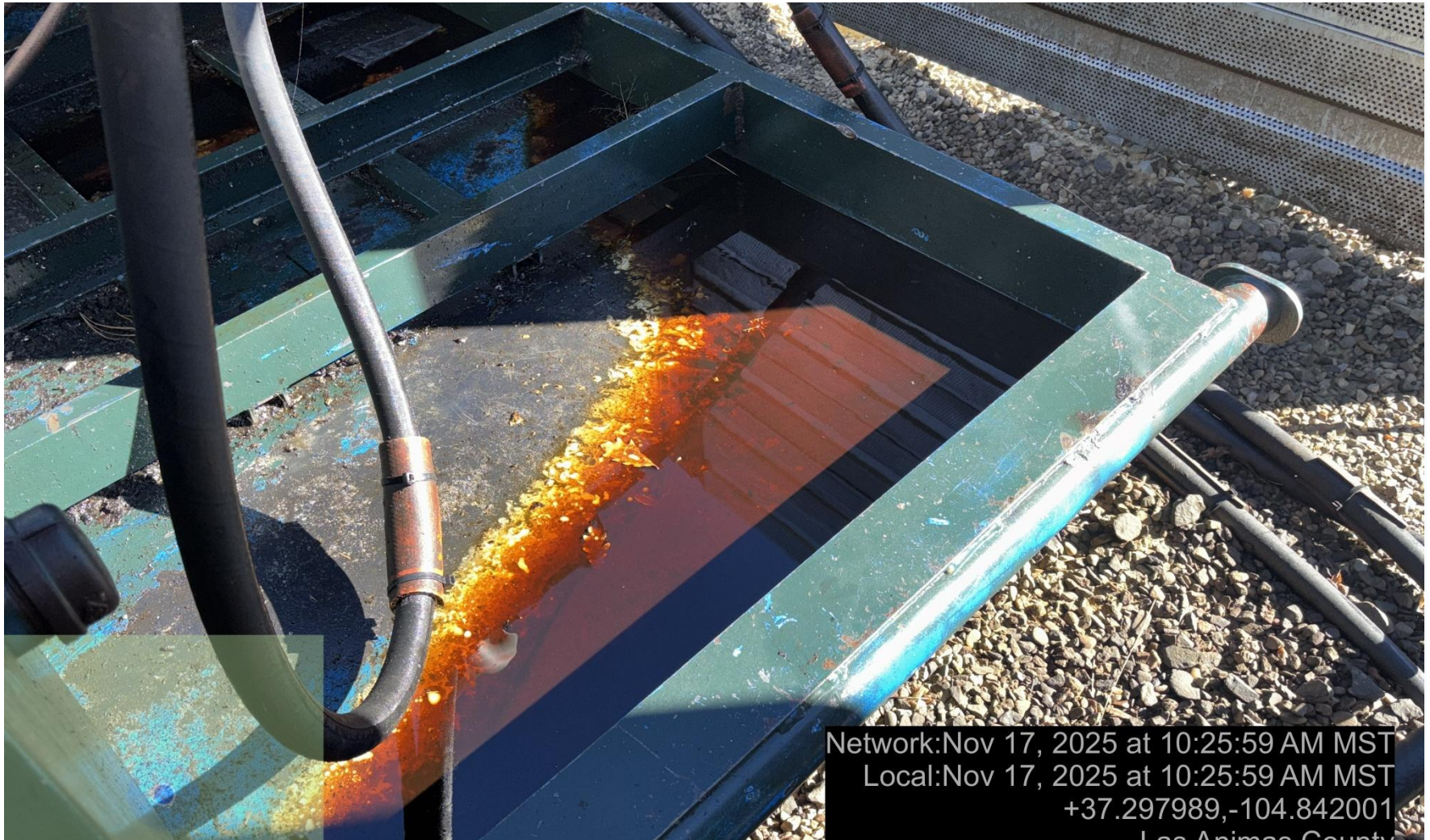
PHOTO 6: OILY WASTE IN PRIME MOVER SKID. DRAIN OILY WASTE REPAIR ALL LEAKS AND REMOVE IMPACTED SOIL PER RULE 1002.(2), D & 1002.f.(2)B, Comply with general provisions of the oil and gas act for wildlife protection AND SB-181 CA DATE 11-18-2025.
