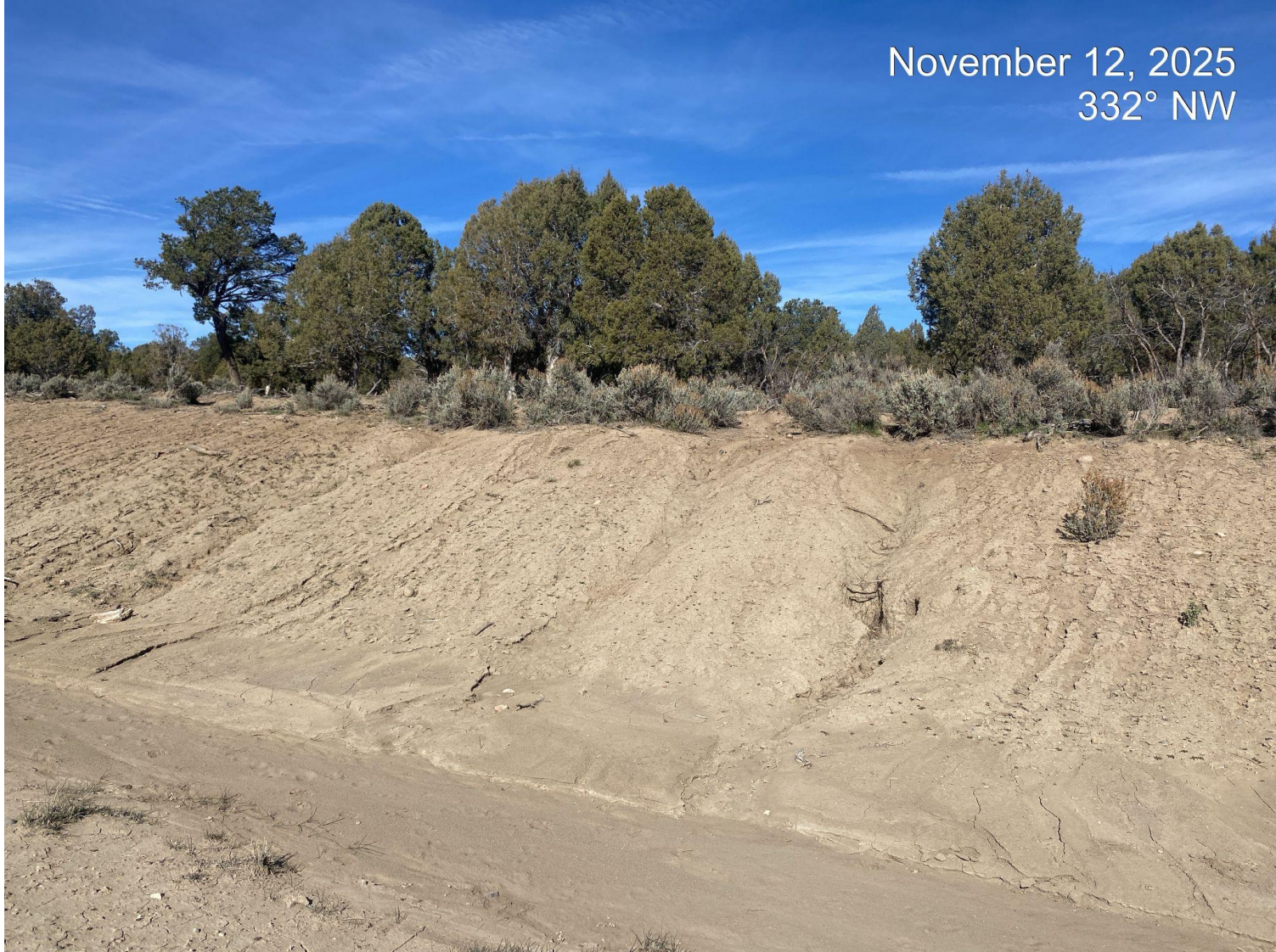
Photo 5. View of gully erosion forming on the location cut slope.
