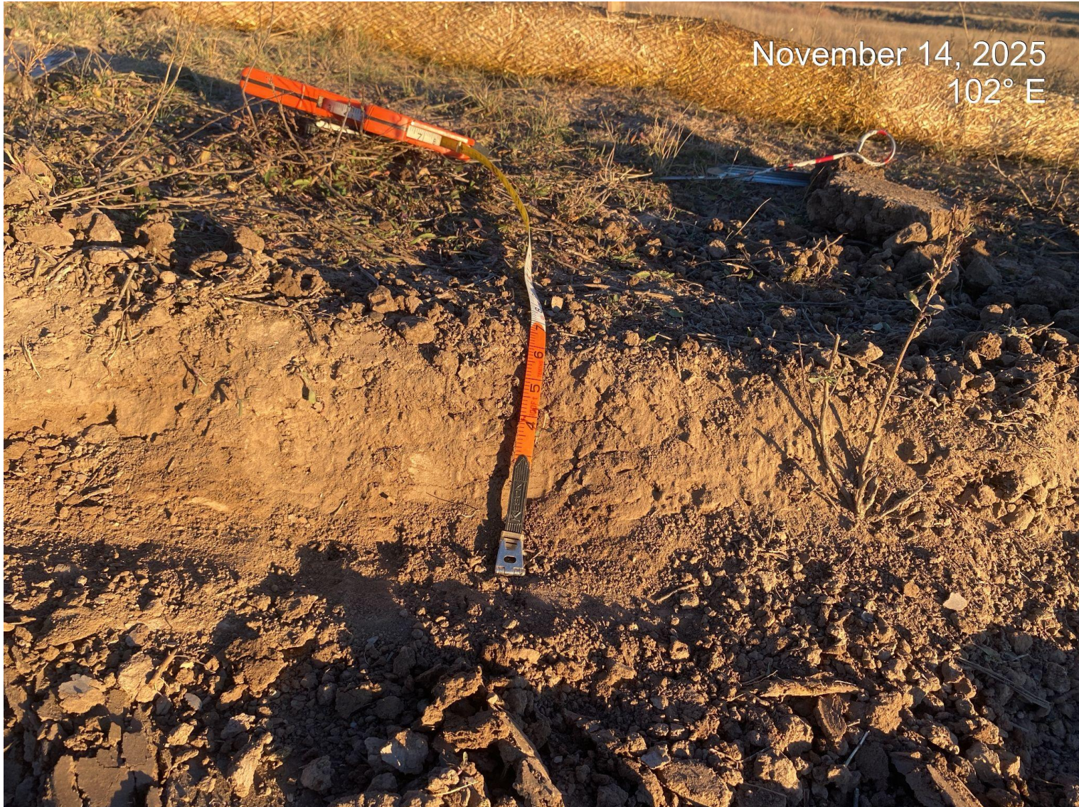
Photo 6. View of cut for topsoil salvage on the location. It appears that the operator is salvaging the 6 inch minimum requirement of topsoil
