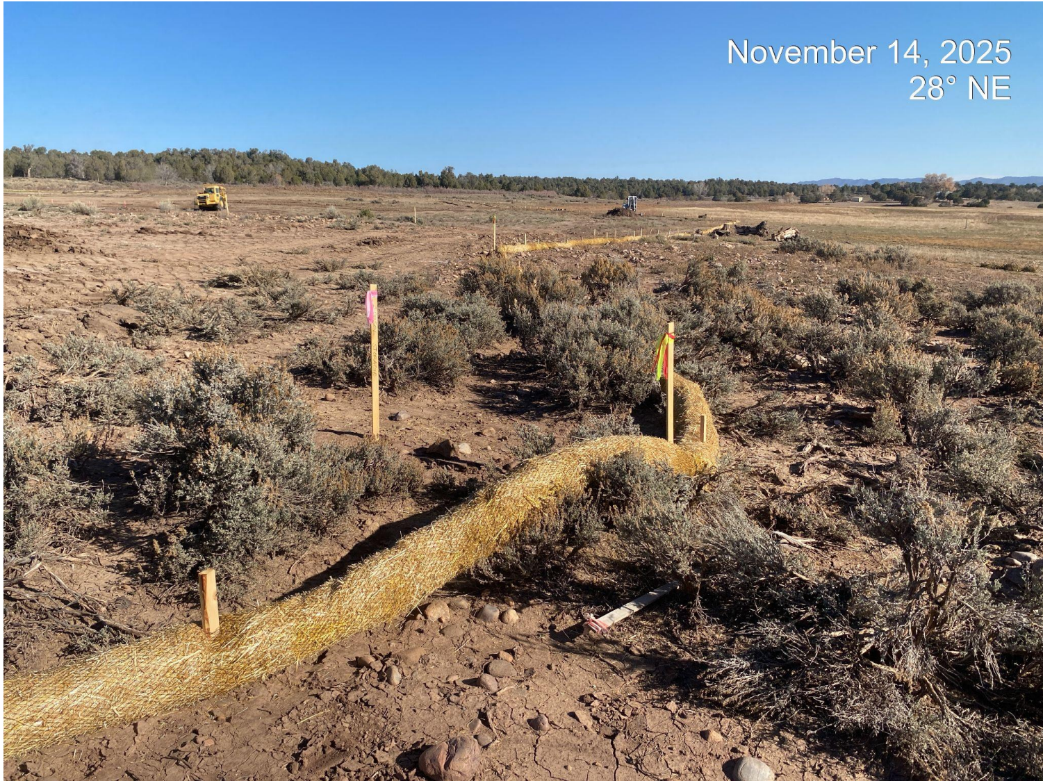
Photo 5. Additional view of perimeter BMP wattles on the southern and eastern edges of the disturbance which have not been installed per good engineering practices (trenched).
