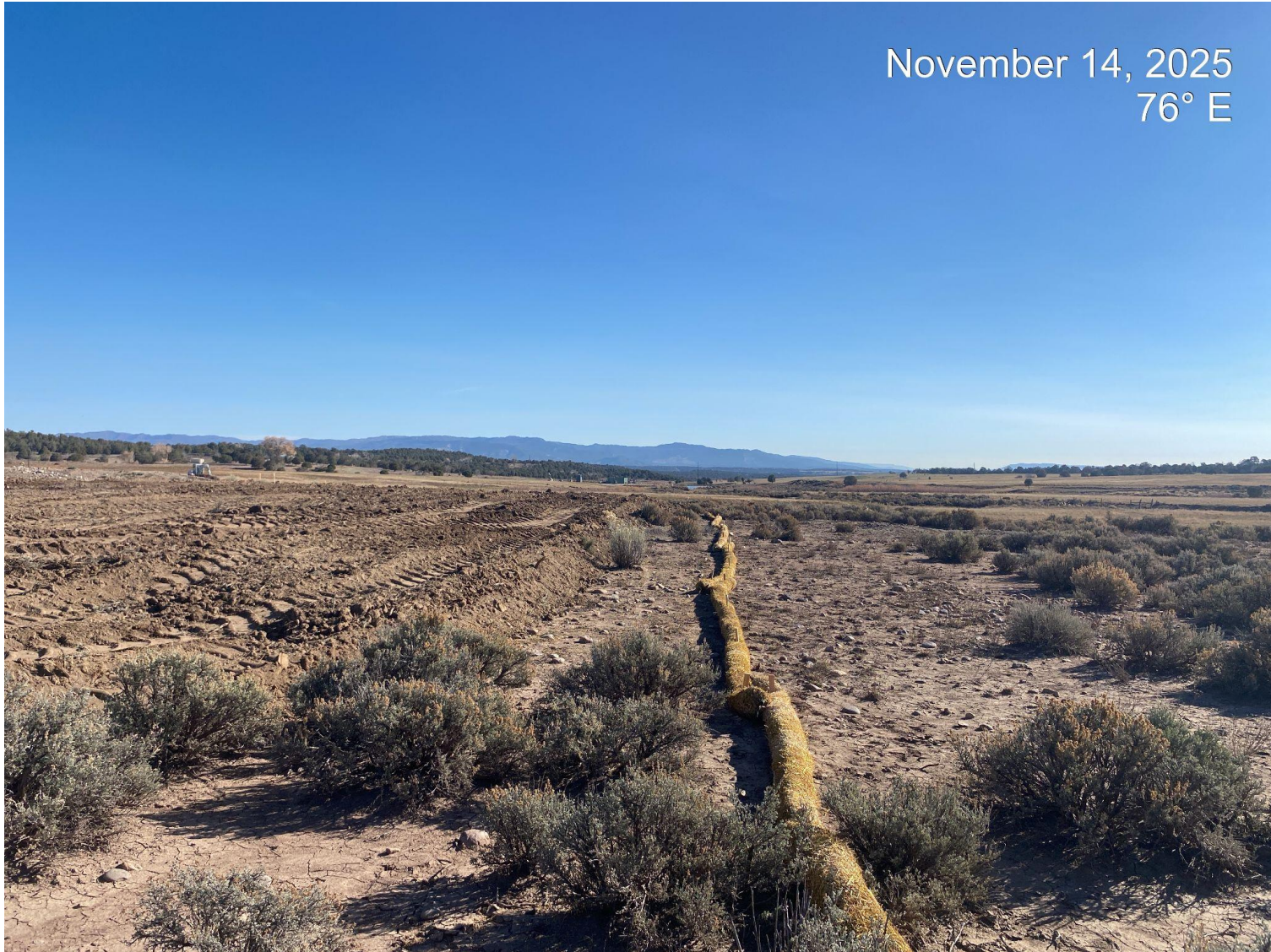
Photo 4. View of the southern edge of the well pad and perimeter BMP wattles. Note: wattles have not been installed per good engineering practices (trenched) in these areas.
