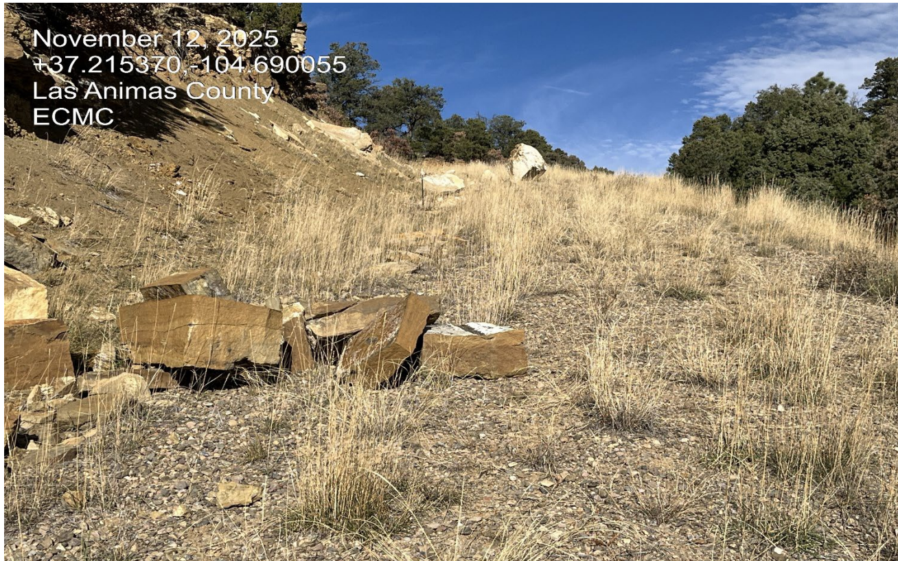
Photo 2. Facing northeast along the access road. There are large boulders that have fallen onto the roadway.
