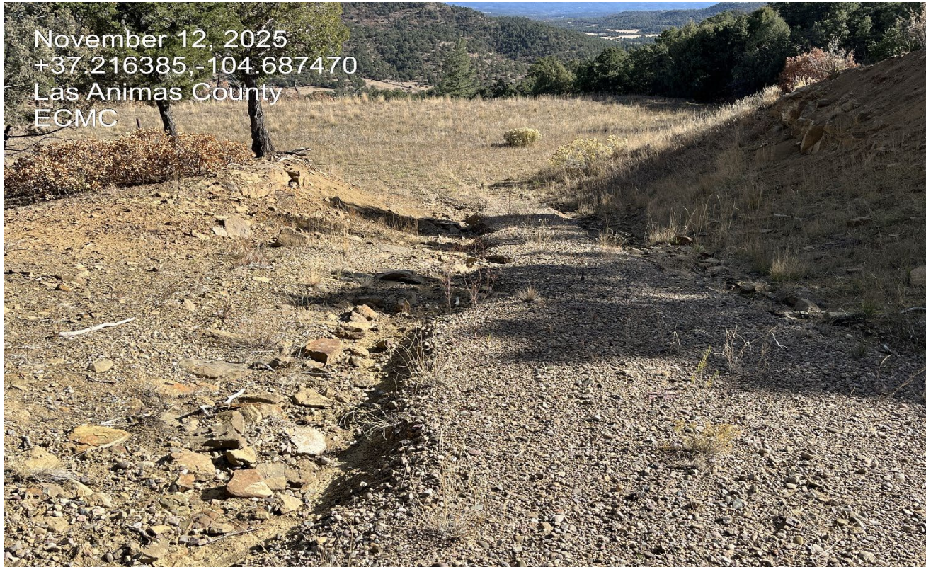
Photo 3. Facing southeast. There is erosion along this last remaining part of the road leading to the location.
