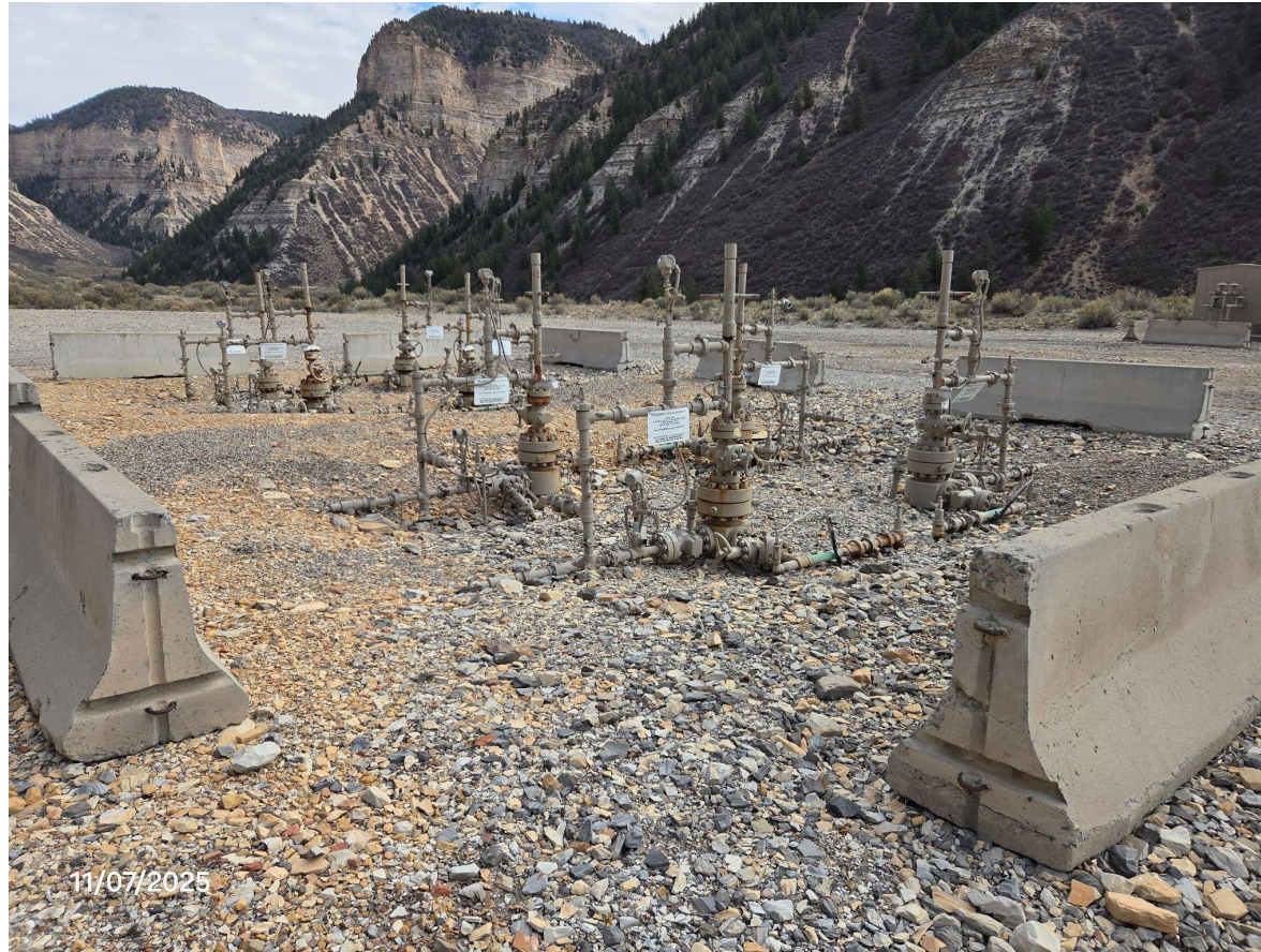
Photo 3: Photo show signs have been installed at the wellheads.
