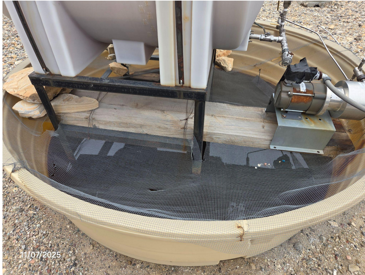
Photo 7: Photo shows fluids spilled within containment.
