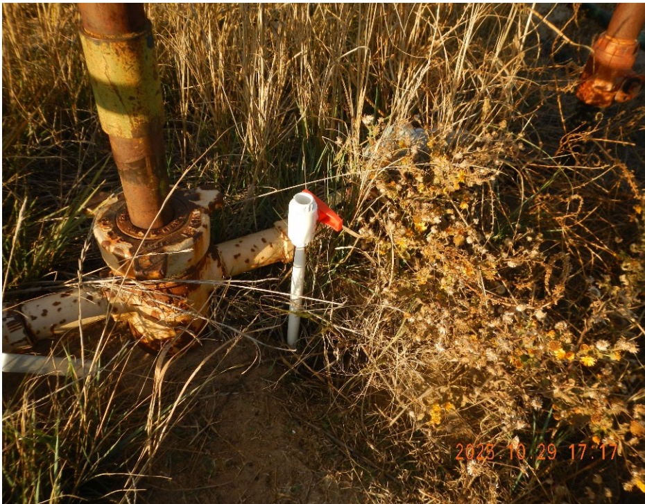
2. View Bradenhead plumbed to surface at wellhead.
