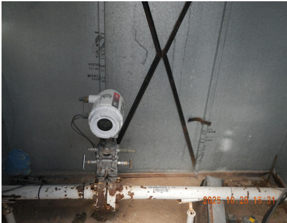
3. Gas Meter inside Meter Shed.
