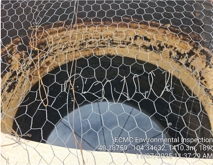
Photo 5 – Oil noted on water in bottom of western produced water tank.
