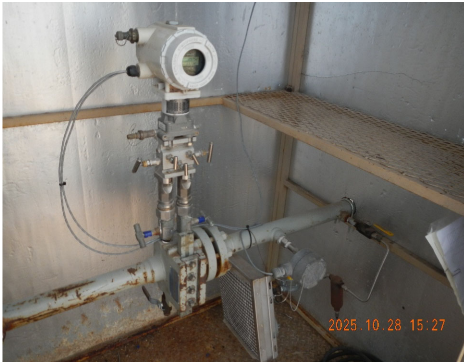
5. Gas Meter inside Meter Shed.
