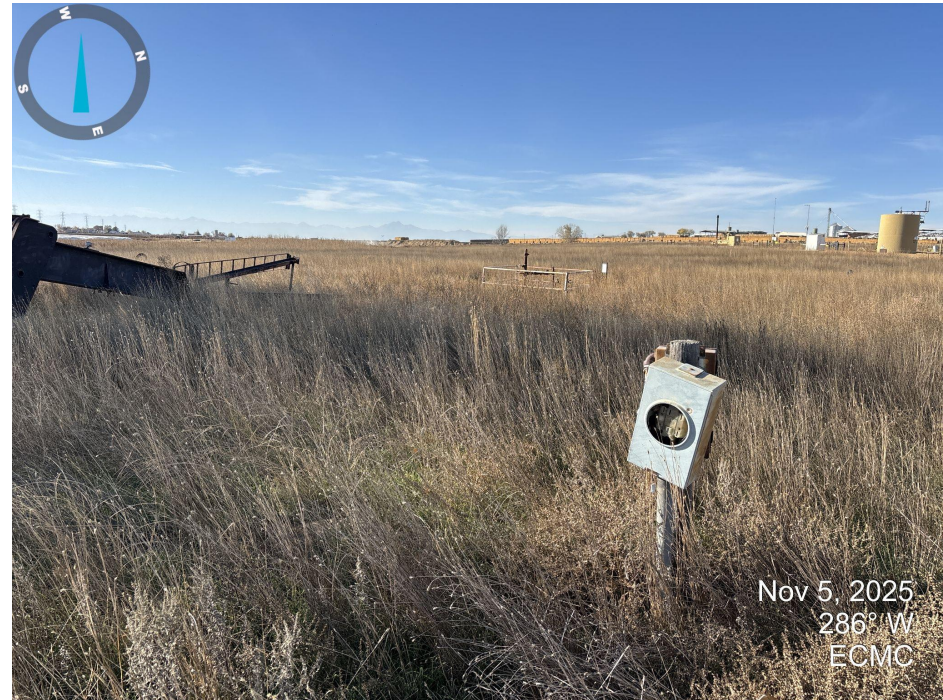
Photo 6. Photo taken on the east side of the location. Unused electrical meter.
