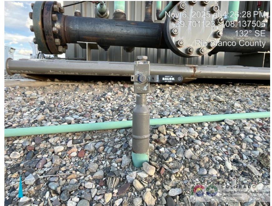
Photo # 3893 Unused flowline lacks lockout tagout (OOSLAT)
