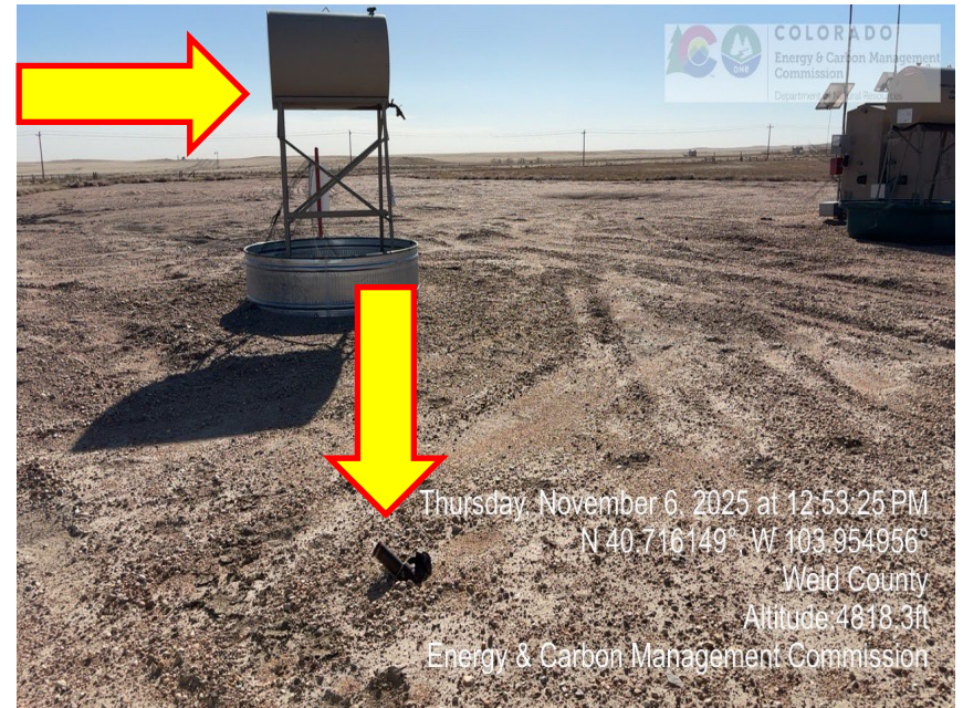
Photo 4 – Unused Pipe and Day Tank
