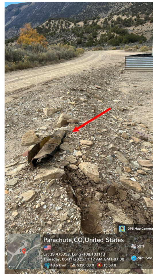
Photo 9 – Trash in and around earthen berm on South side of Tank Battery
