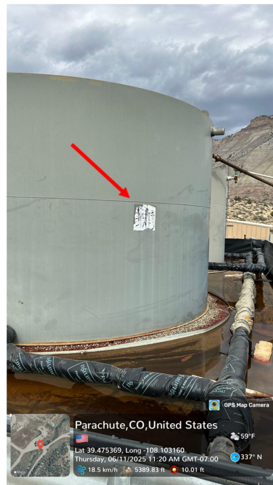
Photo 6 – Signage on tank, facing North from Southeast corner of Battery
