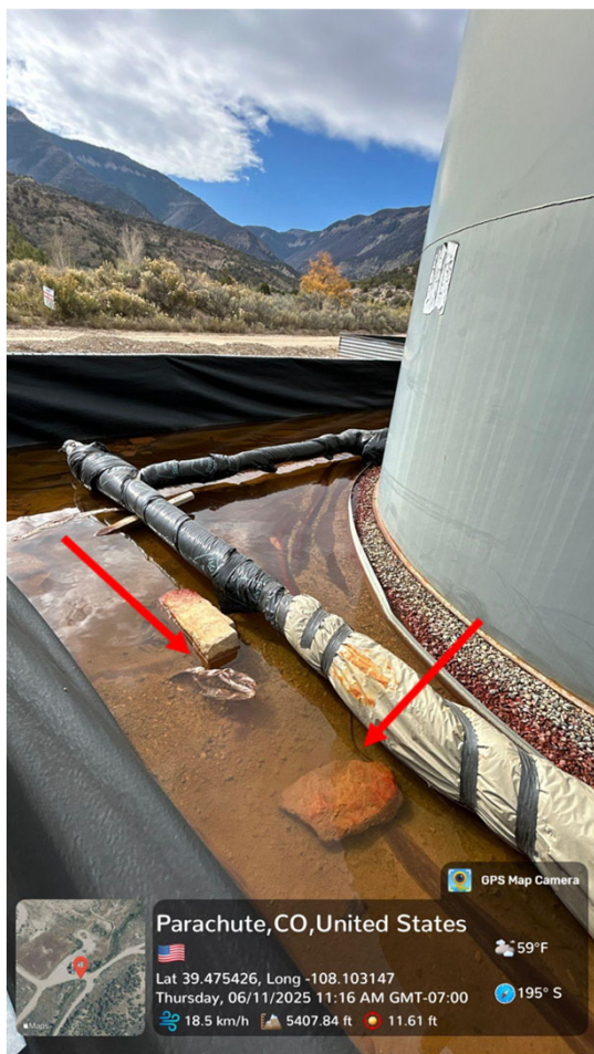
Photo 5 – Rocks, debris, and standing water on liner in containment area
