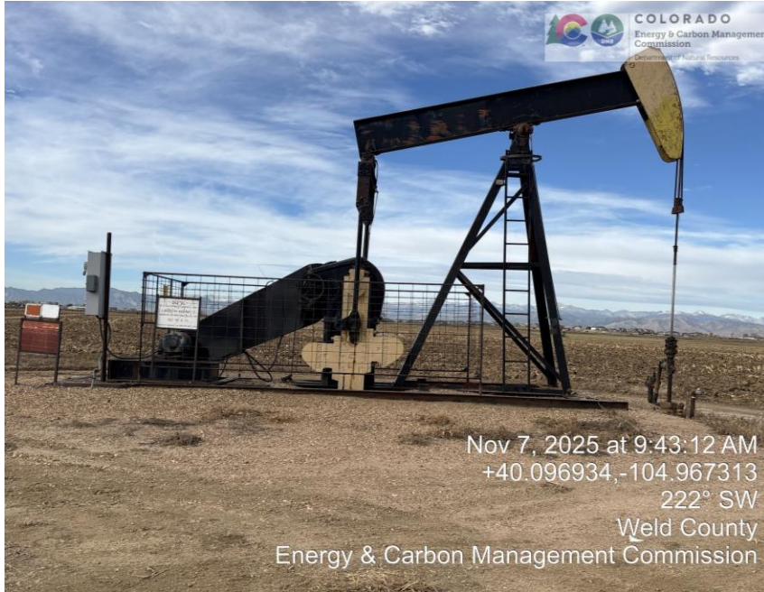
Photo 1 well head and equipment
