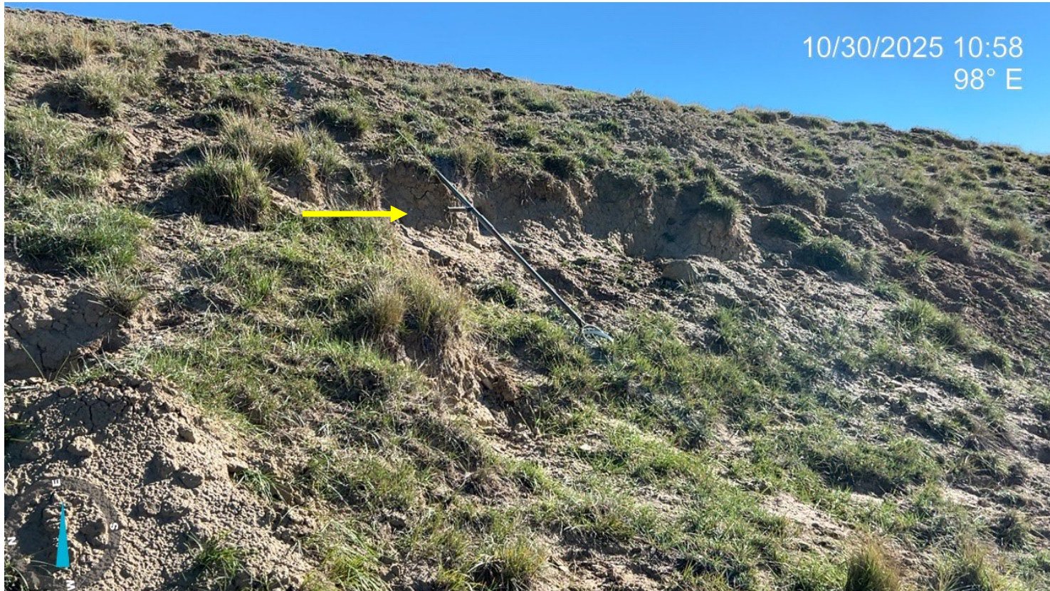
Photo 6: Photo showing pipe debris that is present on the eastern cut slope and requires removal.
