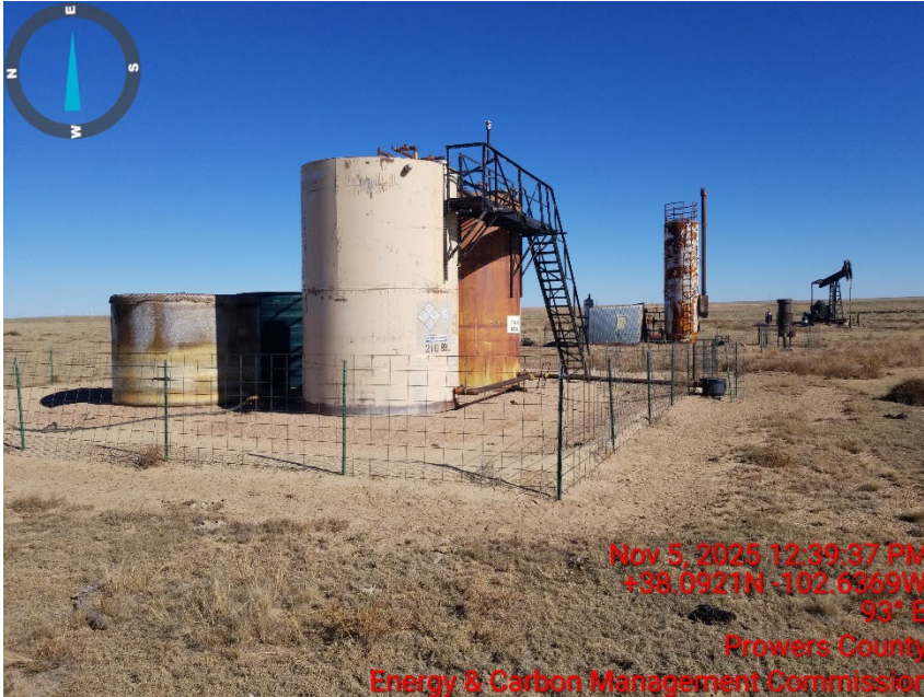
3. Labeling on tanks are missing
