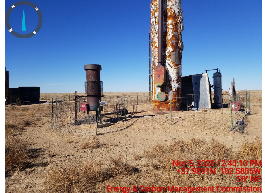
4. Treater, ECD and VGS. Misc debris inside the fence needs removed
