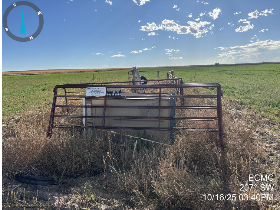
Photo 1. Photo taken of the well location, facing southwest. Photo illustrates that fencing is stacked on the location and a porta potty is laying on its side.
