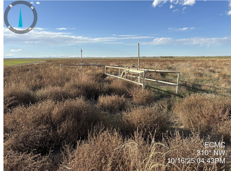
Photo 6. Photo taken of the tank battery location, facing northwest. Photo illustrates that midstream equipment remains on the location and final reclamation does not meet Rule 1004 standards as weedy annual vegetation was observed across the location.
