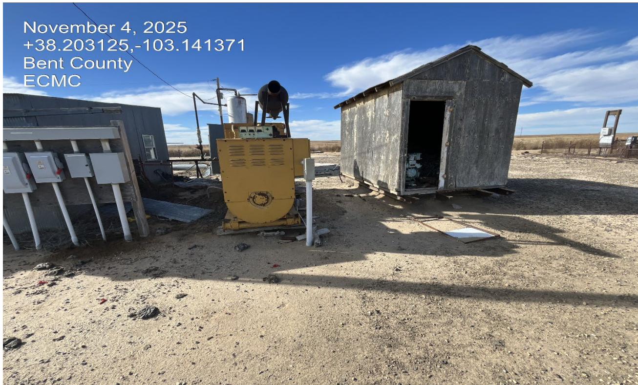
Photo 6. Facing west at center of location. There is a birds nest inside the sheds which are in disrepair.
