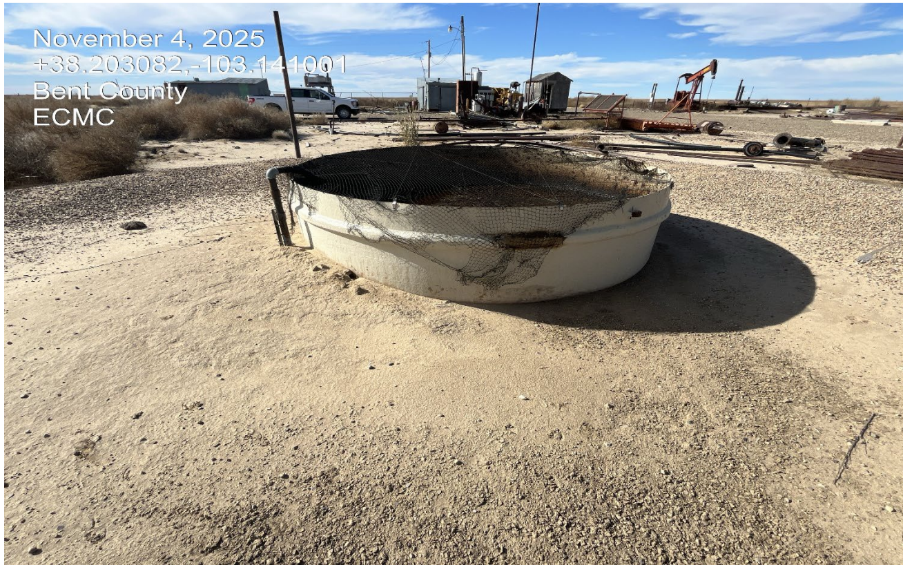
Photo 14. Facing east at the south side of the location. This open top tank remains with oily fluids. Wildlife netting is installed.
