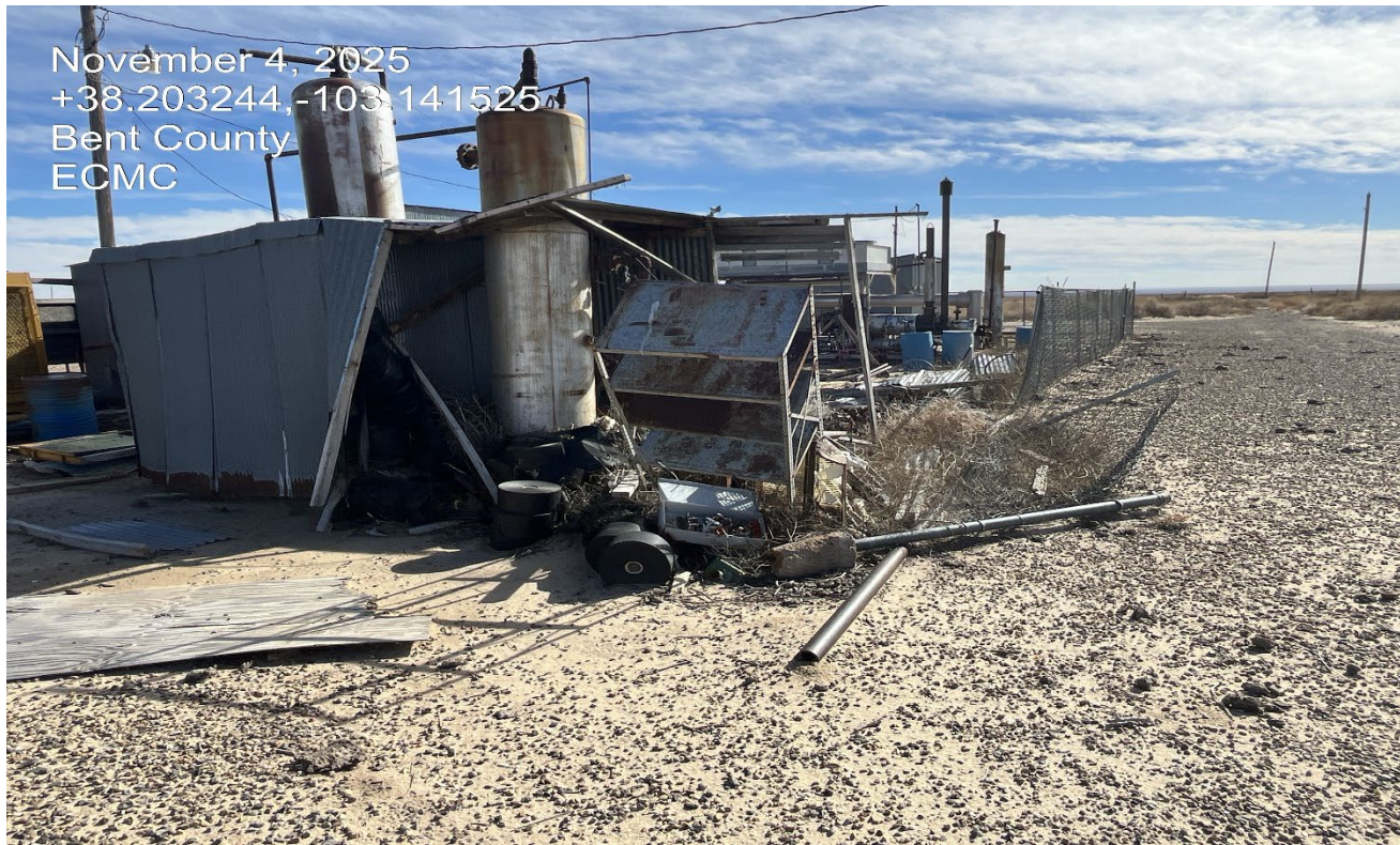
Photo 8. Facing southeast at the west side of the location. This shed and fence are in disrepair with supplies have fallen out of the dilapidated shed.
