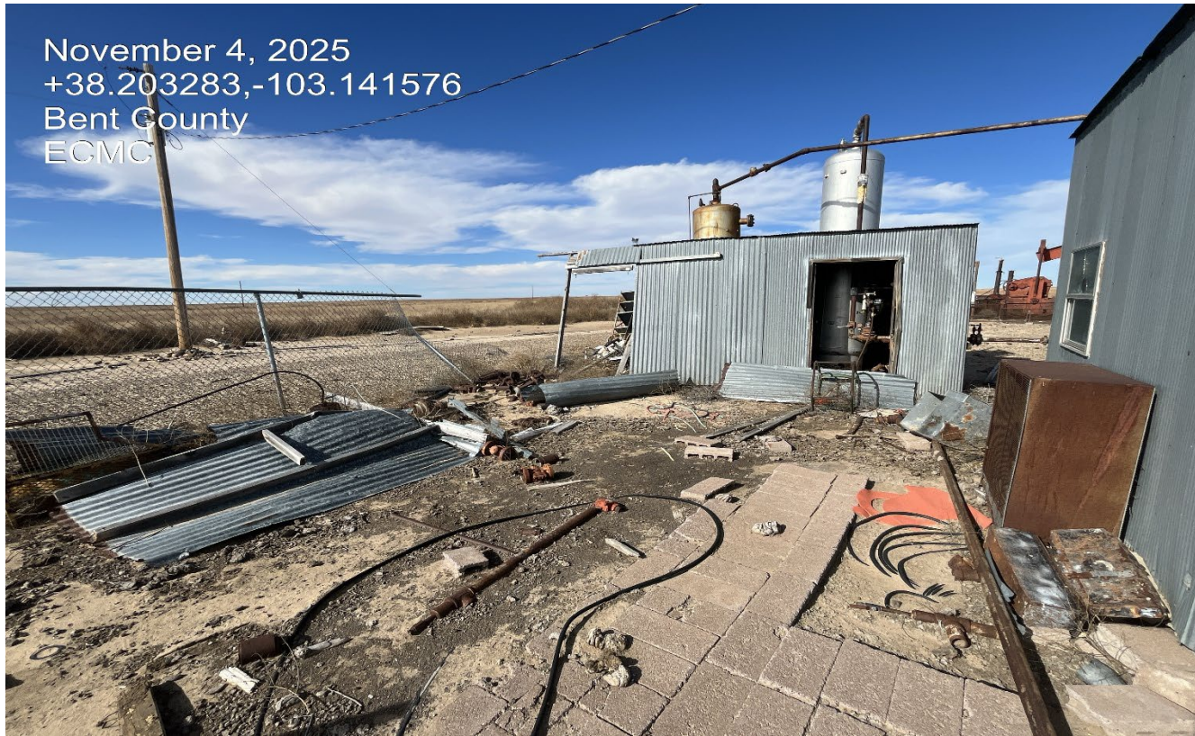
Photo 5. Facing northwest at the sheds and equipment which are in disrepair.
