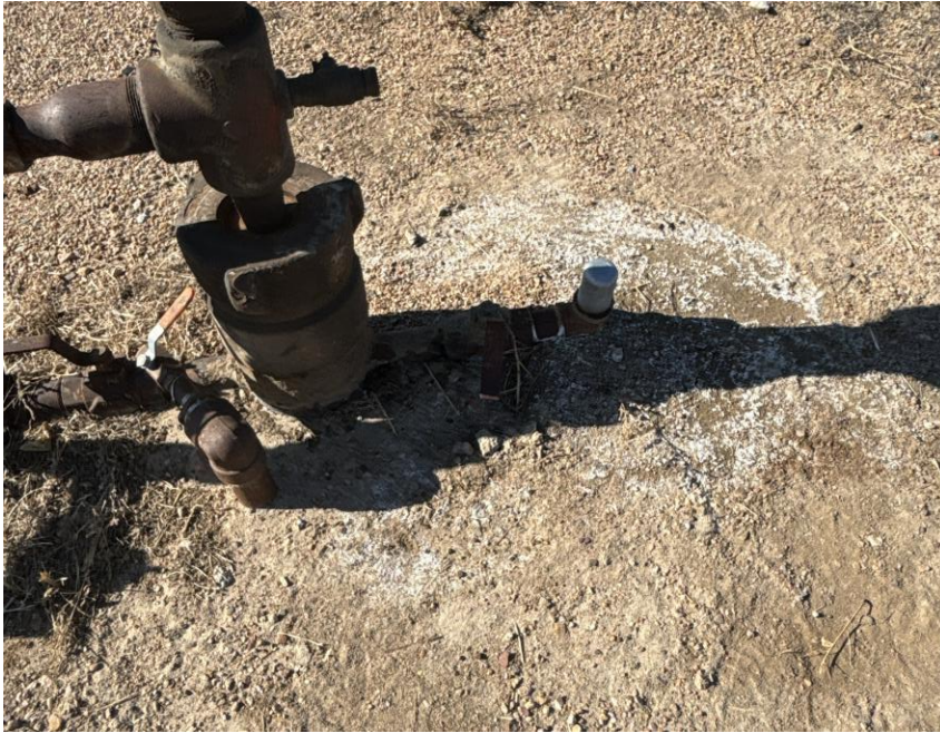
Photo 3 suspect leak at well head
