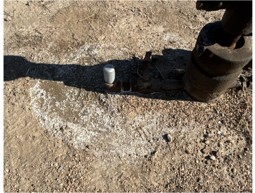
Photo 4 suspect leak at well head
