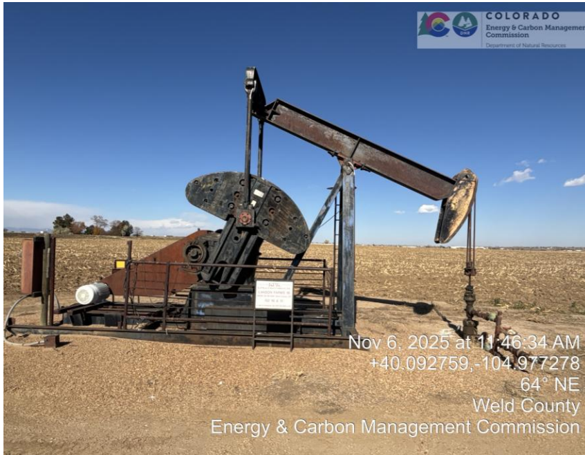
Photo 1 well head and equipment
