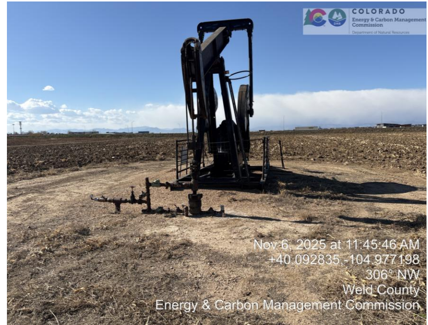
Photo 2 well head and equipment
