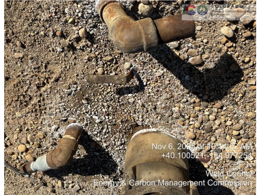
Photo 4 well head area of suspect leak
