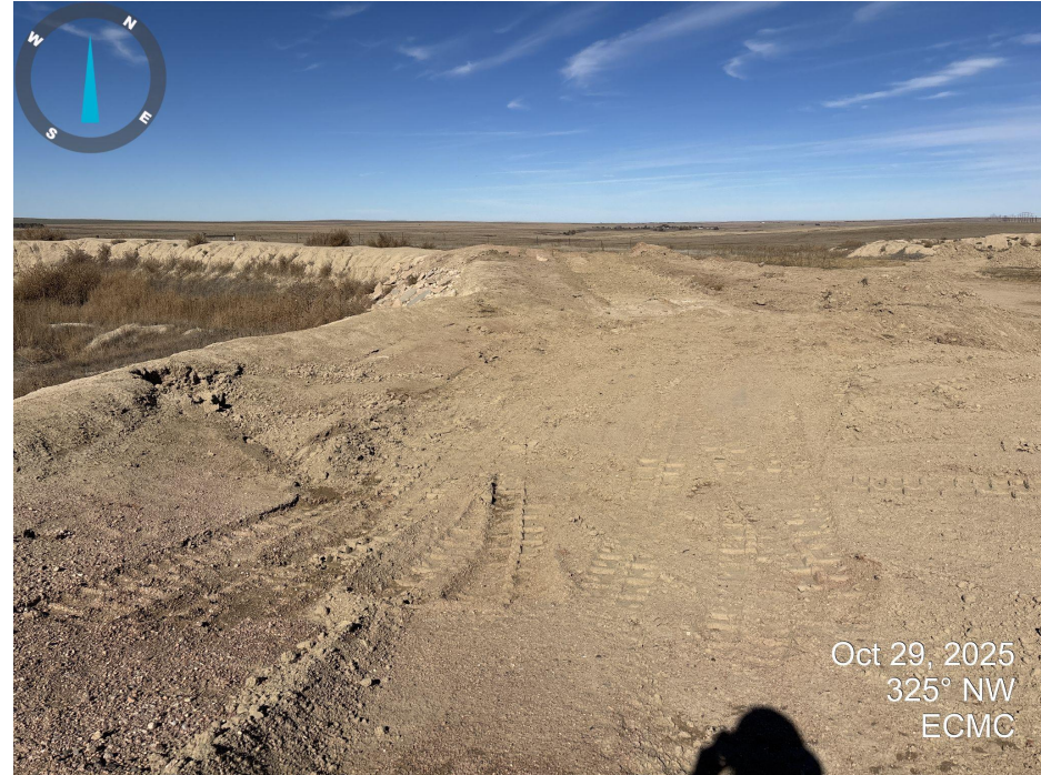
Photo 2. Looking northwest across the former storage tank area. Tanks have been removed. Wooden or cement foundation remains where the former blue open top tank was located.
