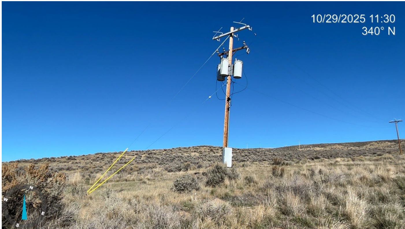
Photo 5: Photo showing an example of utility equipment on and leading to the location that requires removal.
