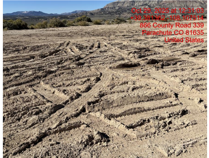
Lack of Stabilization – Photo #01297
