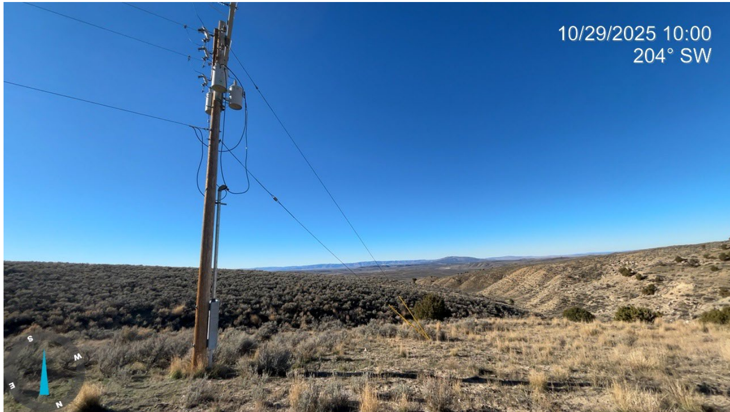
Photo 6: Photo showing an example of utility equipment on and leading to the location that has not been removed.
