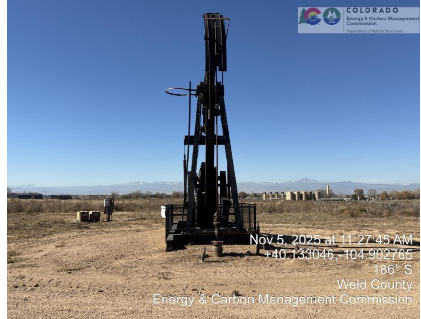
Photo 2 well head and equipment
