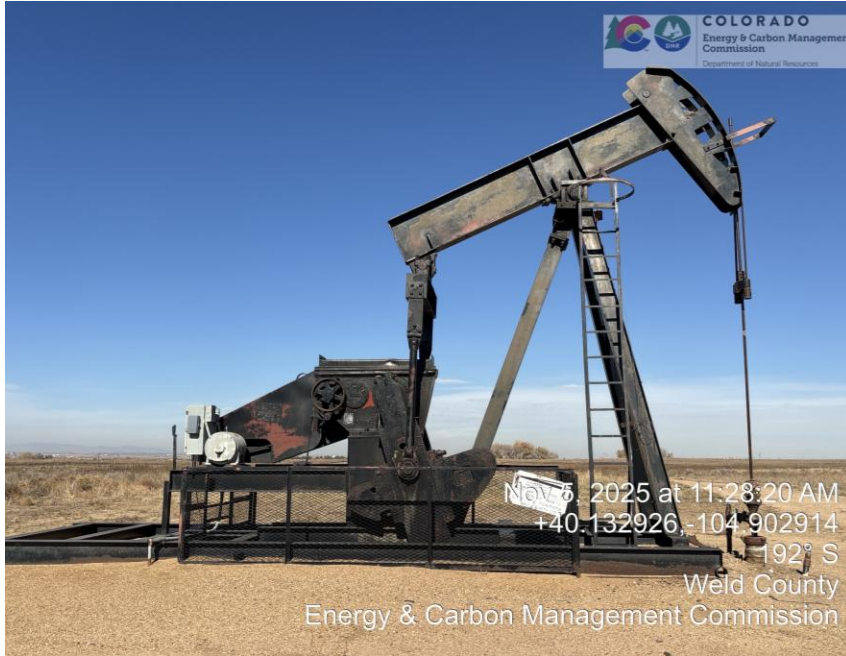
Photo 1 well head and equipment
