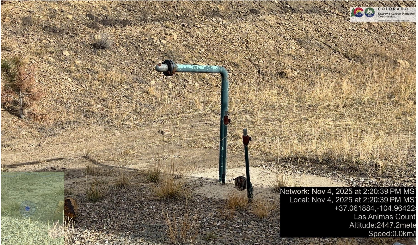
PHOTO 4: UNUSED EQUIPMENT (1-2" RISER AND 1-1" RISER NEAR METER HOUSE). REMOVE OR MARK UNUSED RISERS PER RULE 606. CA DATE 11-14-2025.
