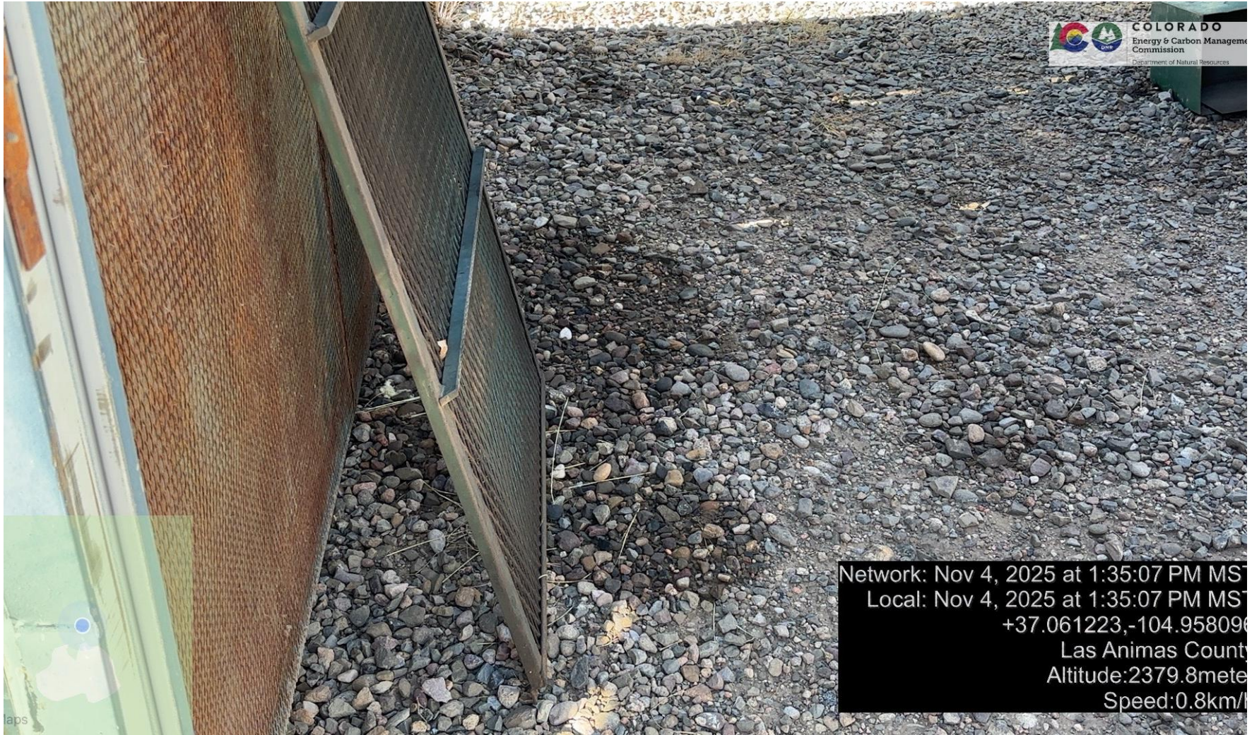
PHOTO 7: MORE IMPACTED SOIL ON SOUTH SIDE OF COMPRESSOR.
