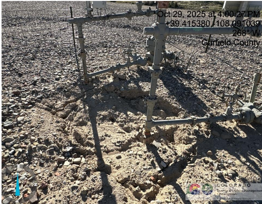
Photo # 4120 Subsidence developing near Williams SG 531-27 wellhead
